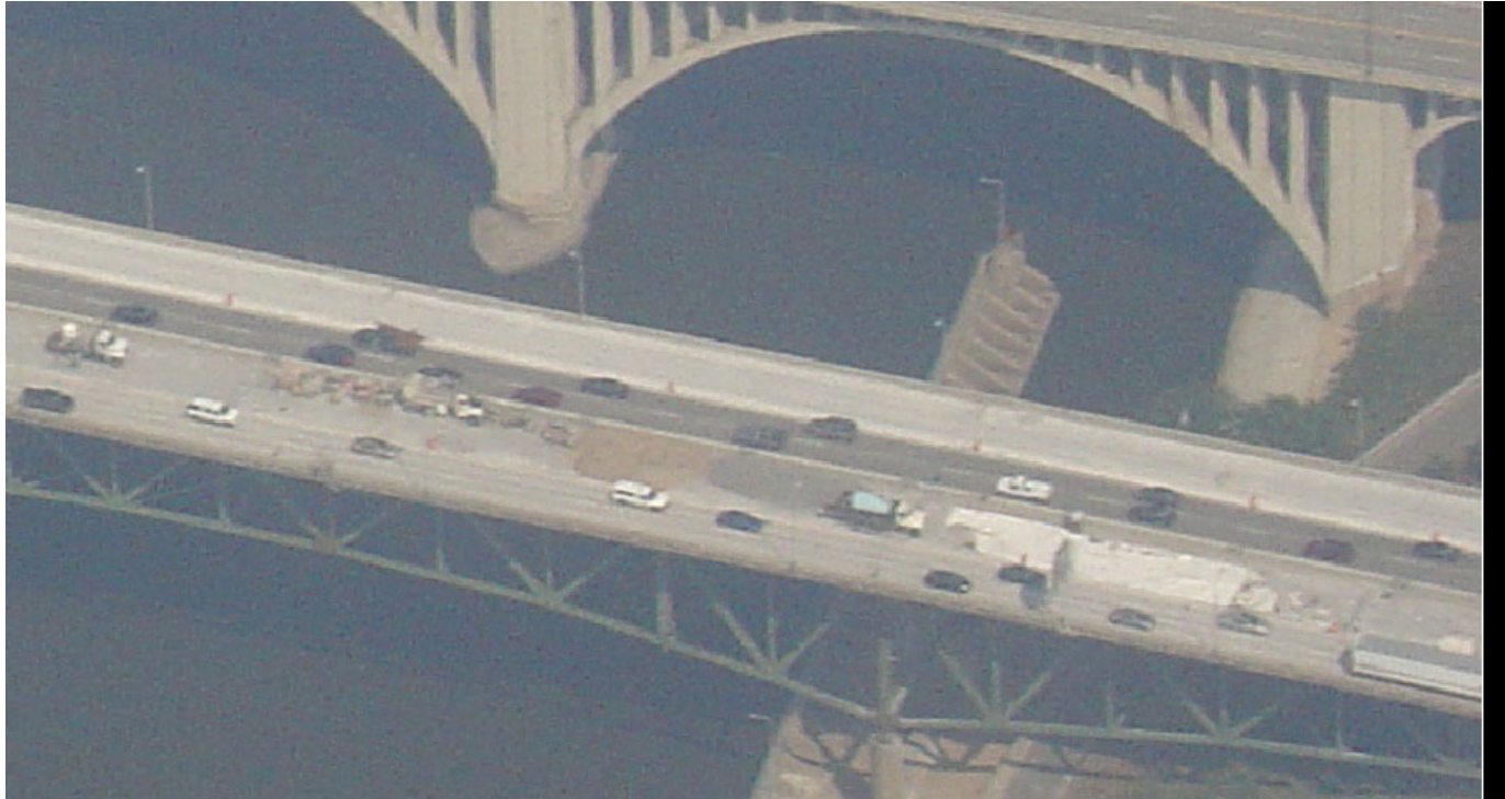
Figure 4. Photograph showing the locations of the aggregate piles on the bridge on August 1, 2007 at 15:47:58 Central Daylight Time.
