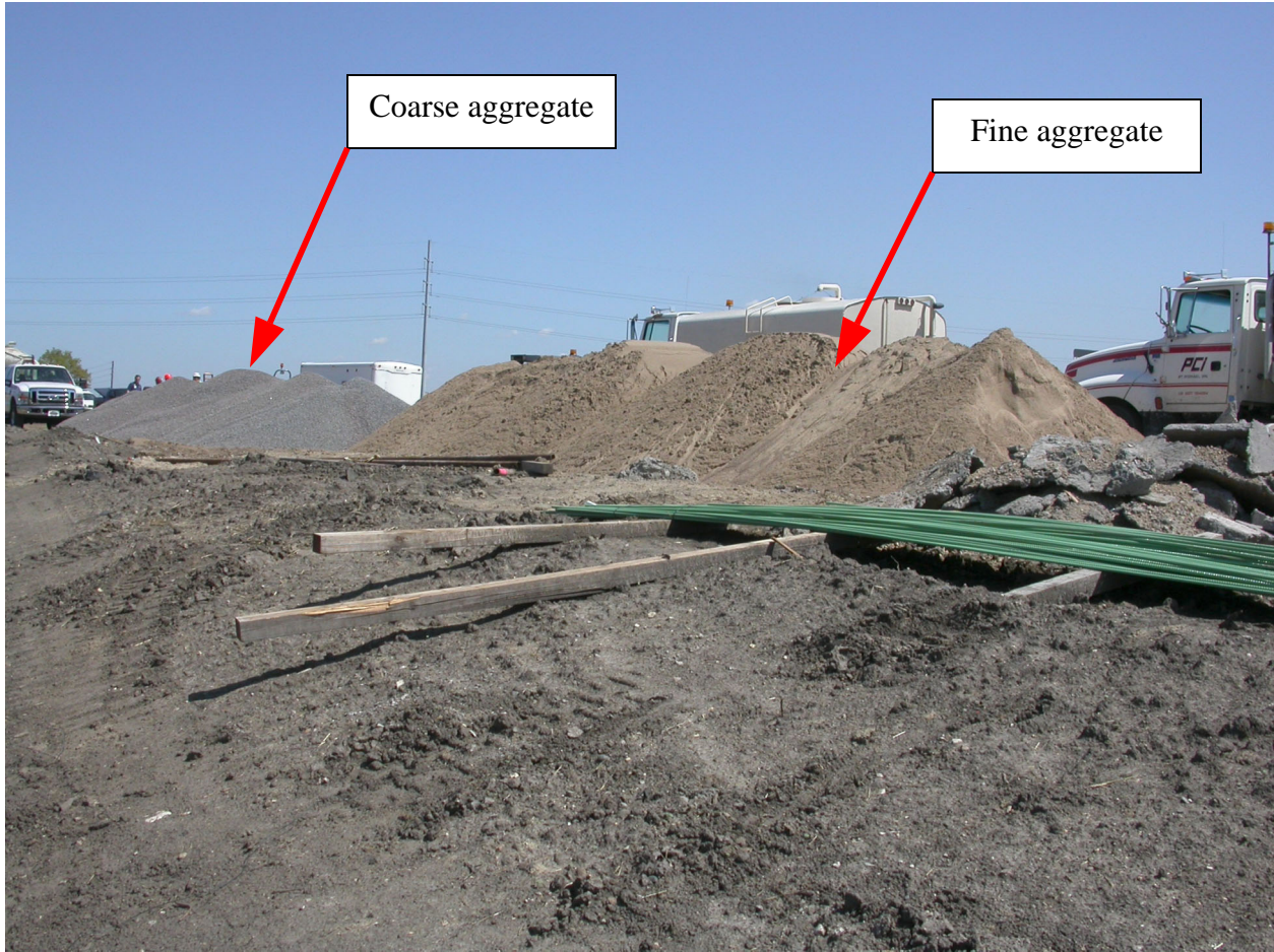
Figure 3. Piles of aggregate delivered to another job site. The quantities of coarse and fine aggregate were similar to the quantities placed on the bridge on the day of the accident. The coarse aggregate pile was approximately 16 feet wide, 60 feet long, and 5 feet tall (at its peak), while the fine aggregate pile was approximately 14 feet wide, 51 feet long, and 6 feet tall (at its peak).
