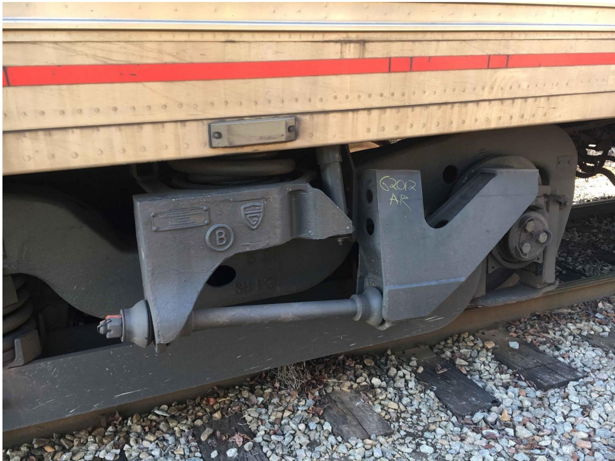
Figure 6. AMTK 62012 Car body truck anchor fixture sheared from side sill (A-End right side).
