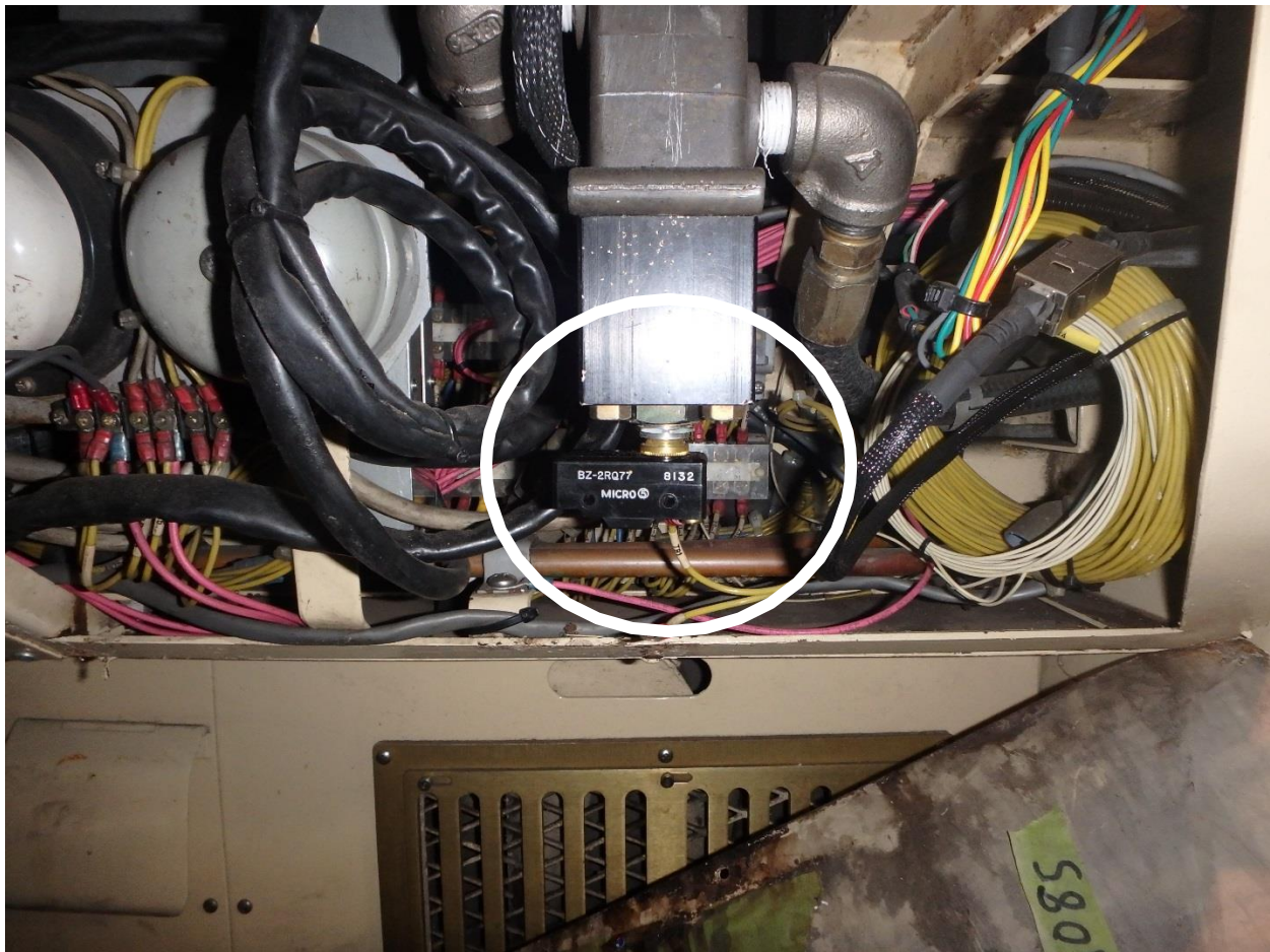
Figure 7. Emergency brake push-button electrical switch installed
