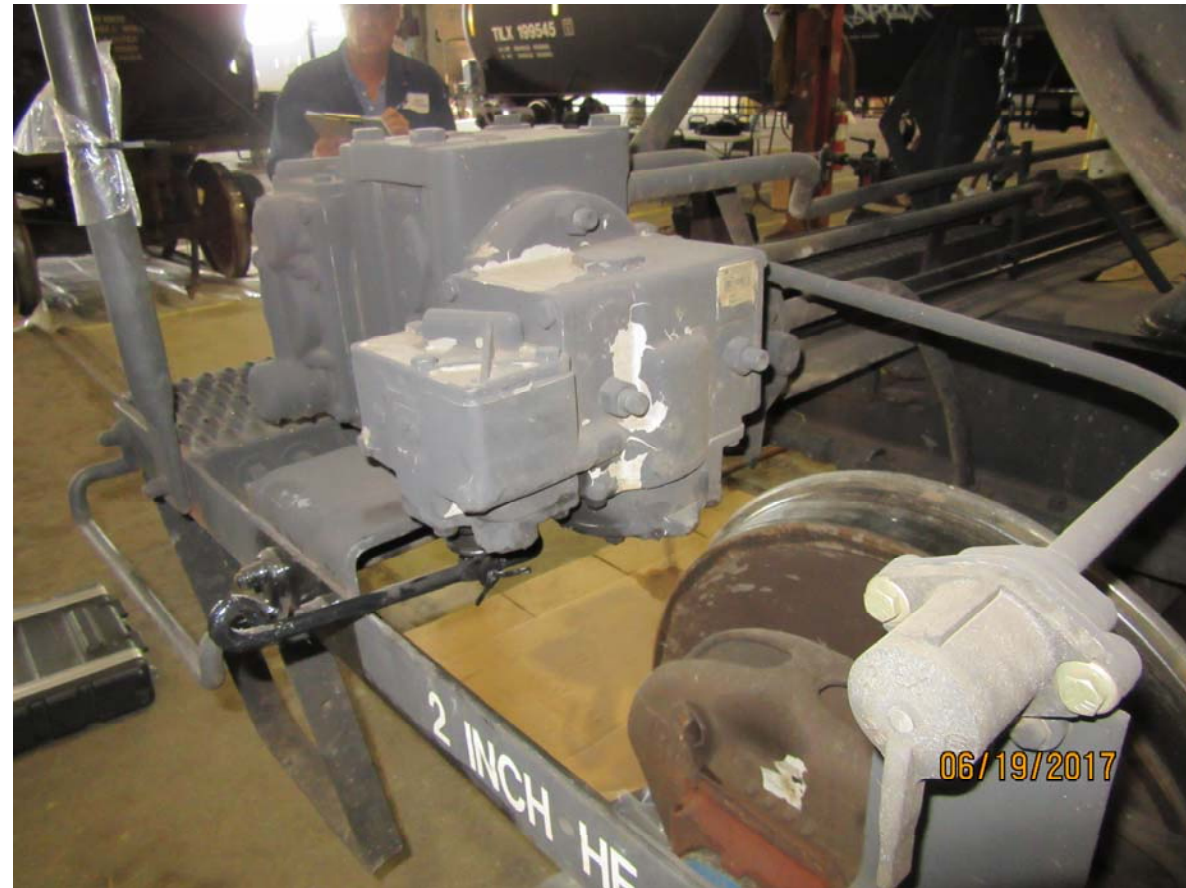
Figure 4266: TILX 198364, brake control valve and brake pipe cut-out valve
