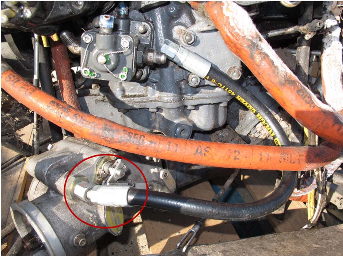
Figure 15. Photograph of unapproved fuel line. The loose connection found on-scene is shown highlighted by the red circle.
