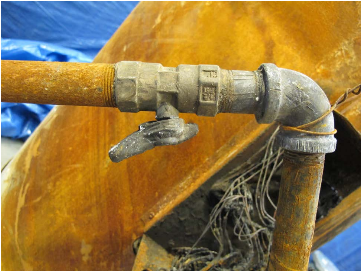
Figure 6. Close-up photograph of manual gas shutoff valve.
