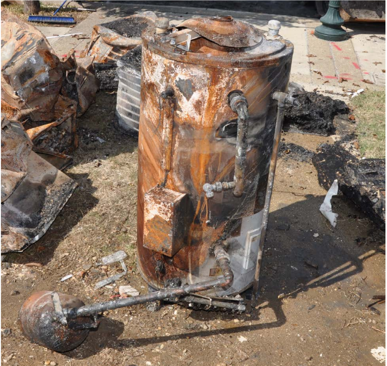
Figure 1. Overall photograph of hot water heater on-scene.
