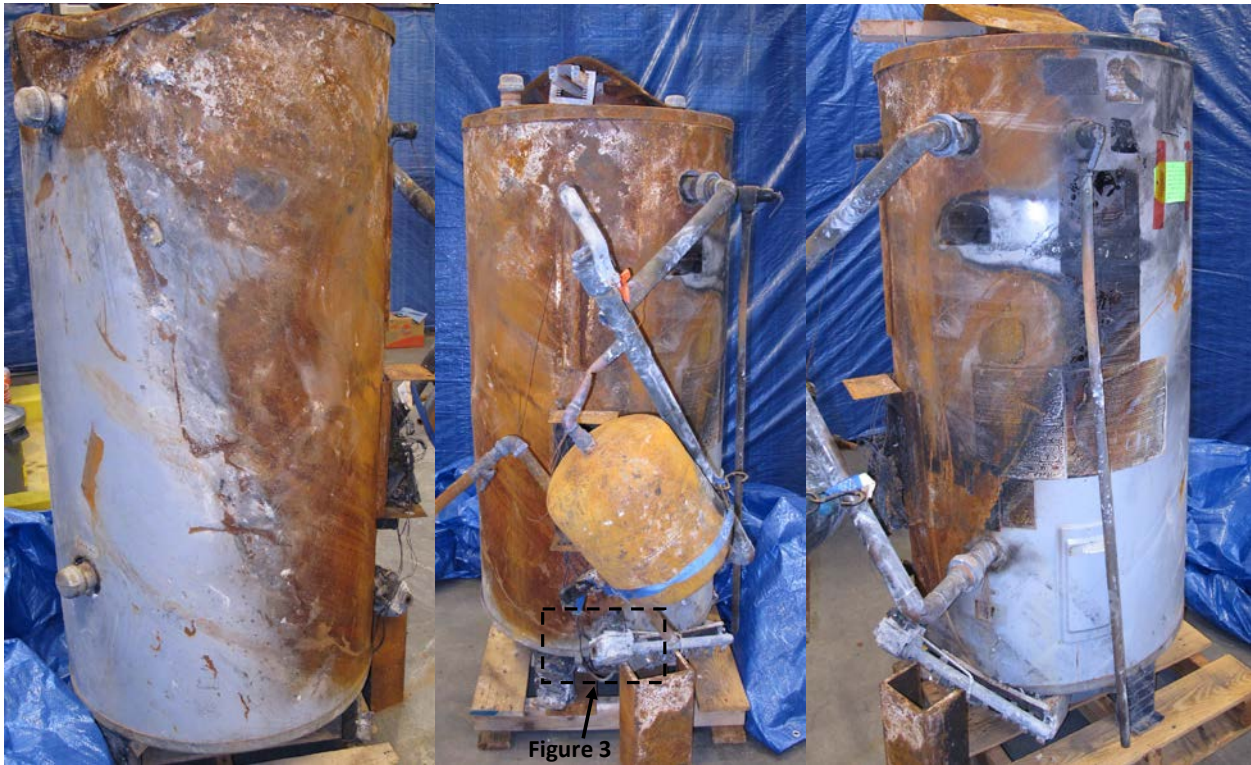
Figure 2. Overall view of thermal damage to exterior of water heater.
