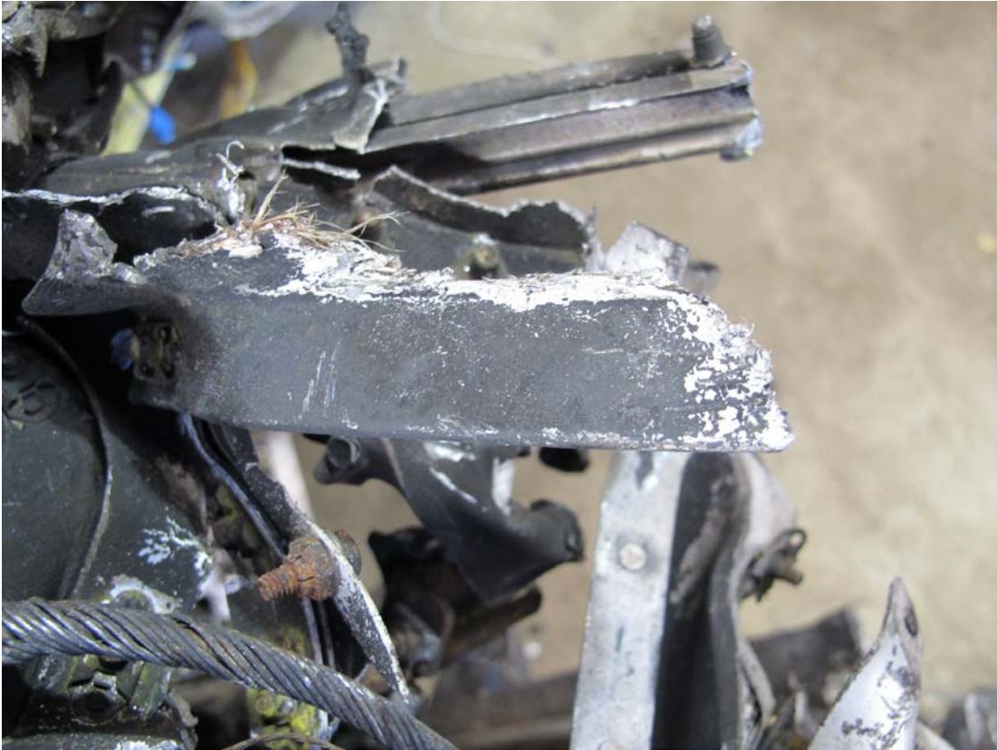
Figure 11. Closeup of broomstraw on structure near main bus tie circuit breaker panel.
