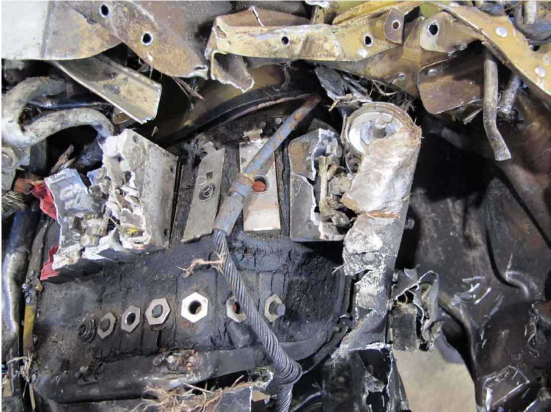
Figure 13. Photograph of underside of main bus tie circuit breaker panel.
