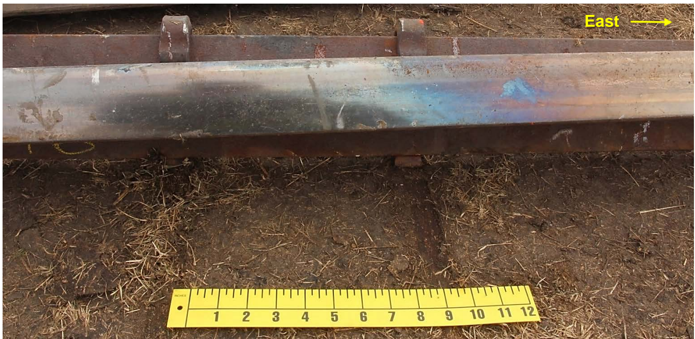
Figure 34 – The middle of the 4S rail piece, showing heat tinting on the head surface (on-scene photo).
