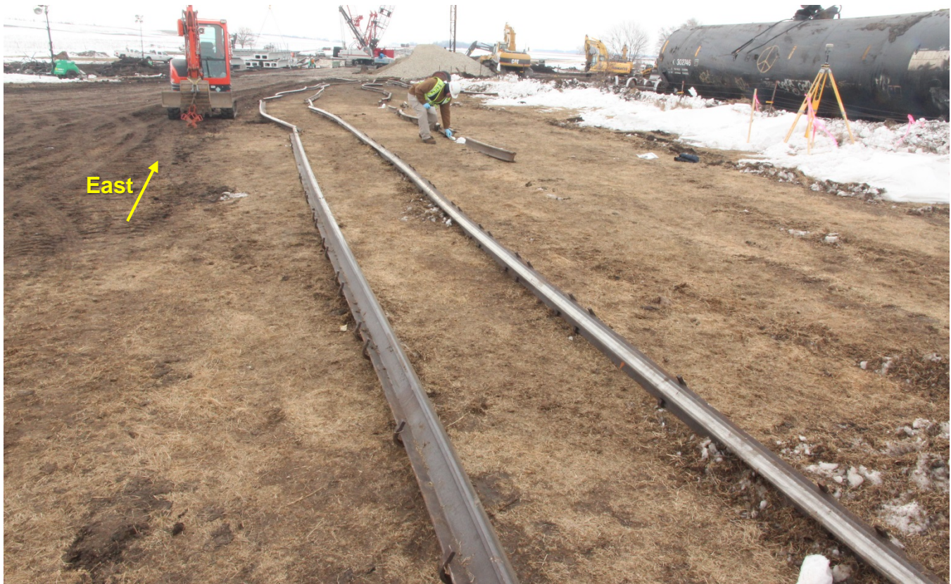
Figure 3 – A view of the rail reconstruction, facing toward the direction the train traveled (east).
