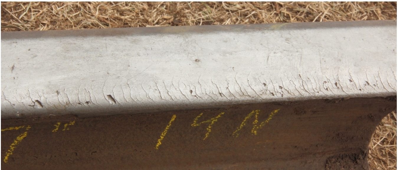
Figure 8 – Closer view of rolling contact fatigue on the gage side of 14N rail section.
