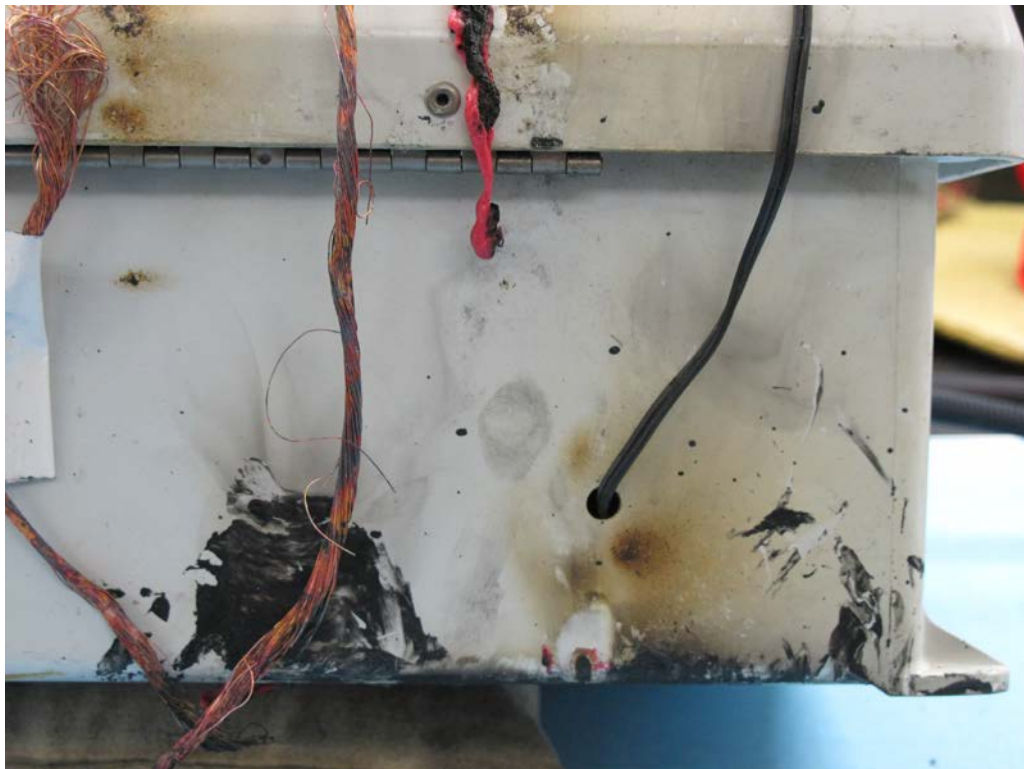
Figure 6. Photograph of lower corner of power distribution box.
