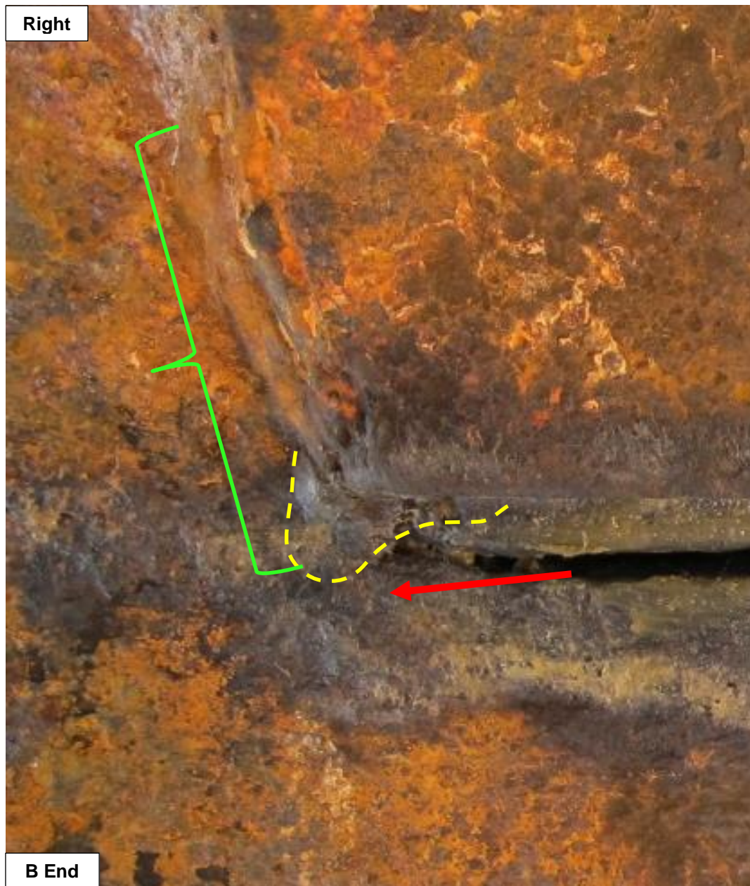
Figure 11. An intact view showing the relationship between the right end (red arrow) of the crack and the nearby right side repair weld (green bracket) with surfaces covered by preservative. The inboard toe of the weld is outlined in yellow.
