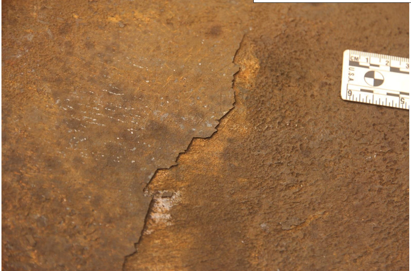
Figure 5. Two views of the surface scaling on the interior of the tank. Broken edges of oxide scale are visible.
