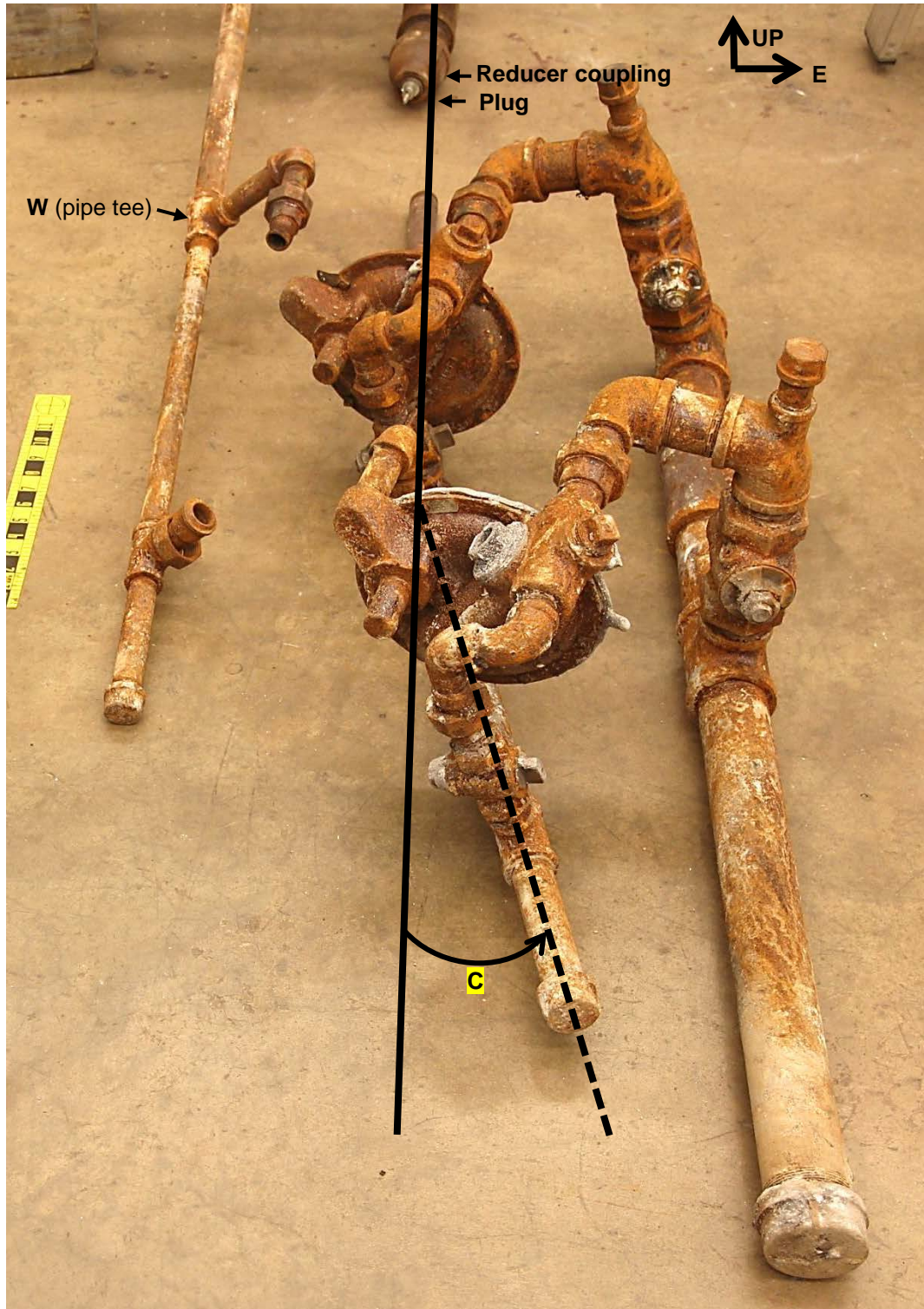
Figure 18. View looking up at the upper and lower pressure regulator assembly.
