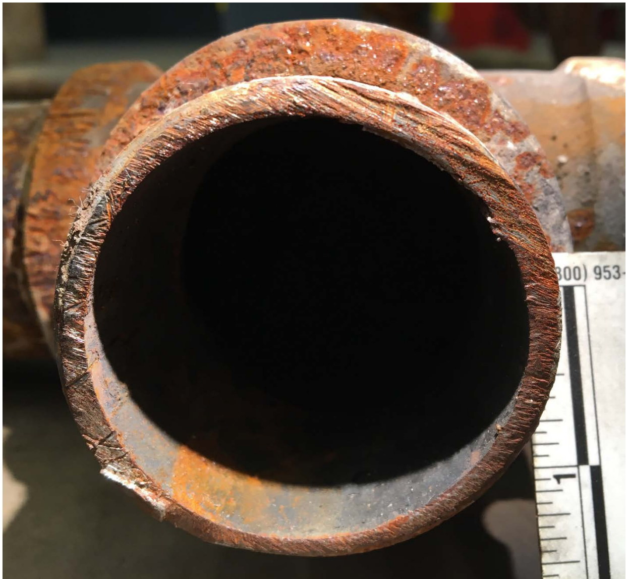
Figure 15. The threaded nipple, indicated by arrow "Q" in figures 1, 2, 13, and 14 that led to a tee for the lower row of gas meters showing saw cut features that extended through the entire diameter.
