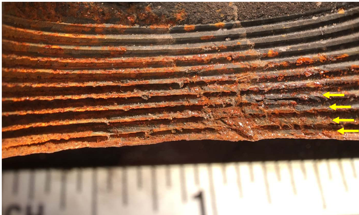
Figure 16. Views looking inside of the pipe tee indicated by arrow "R" in figures 1, 2, 13, and 14 that leads to the upper row of gas meters. Photograph at the bottom of the page shows the diametrically opposite side. The first four threads adjacent to the opening in the areas indicated by arrows exhibited thread deformation damage.
