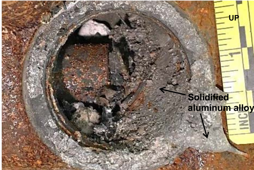
Figure 10. View through the 2-inch diameter side port of the upper gas regulator assembly showing solidified aluminum alloy that encased the orifice and disc portions.
