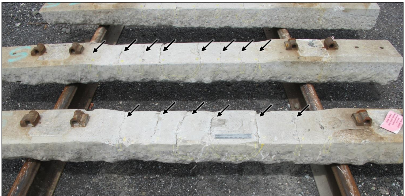
Figure 2. Middle portions of ties S3 and S4 showing multiple transverse cracks as indicated with arrows.
