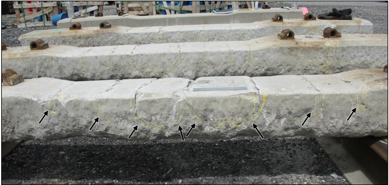
Figure 3. View of the south faces of ties S3 and S4 showing crack features outlined with yellow paint as indicated with arrows on tie S3.
