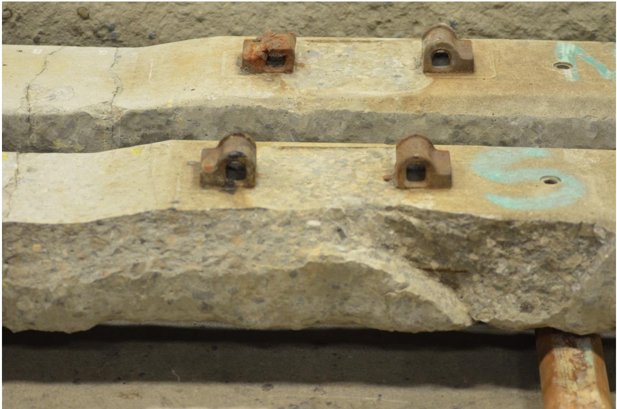
Figure 7. View of freshly broken off concrete area on Specimen S4.
