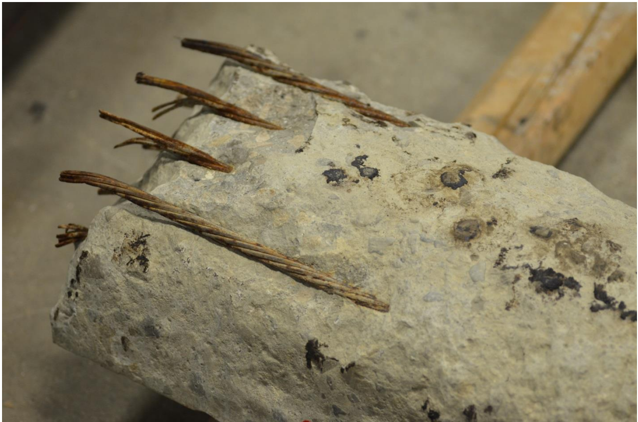
Figure 5. Example of abrasion typically observed at the ends of the railroad ties that sit at the higher elevation side of the curve (Specimen S3).
