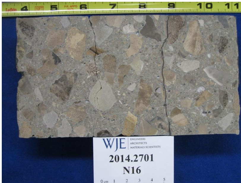
Figure 6. Core N16. Lapped cross section illustrating the appearance of the concrete. In-service top end is on left.
