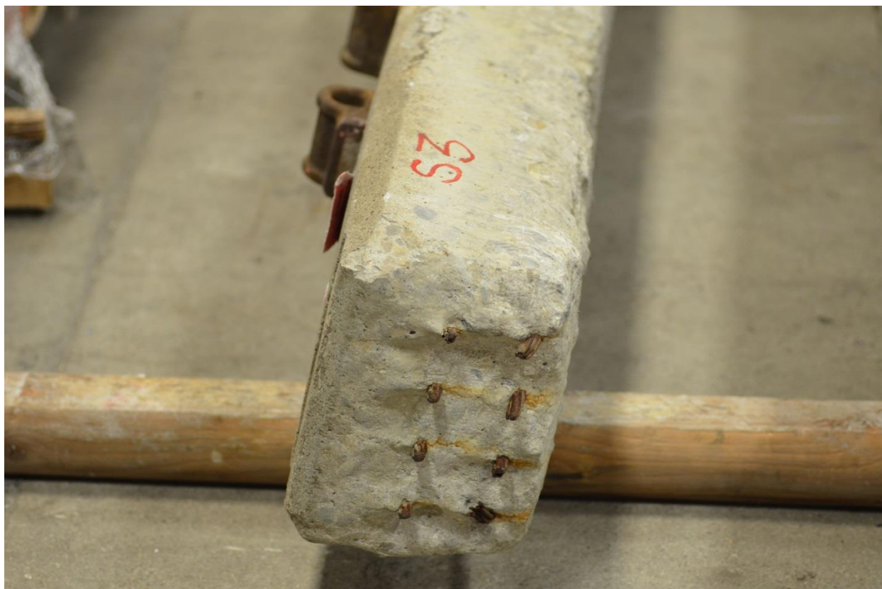
Figure 4. Example of abrasion typically observed at the ends of the railroad ties that sit at the lower elevation side of the curve (Specimen S3).
