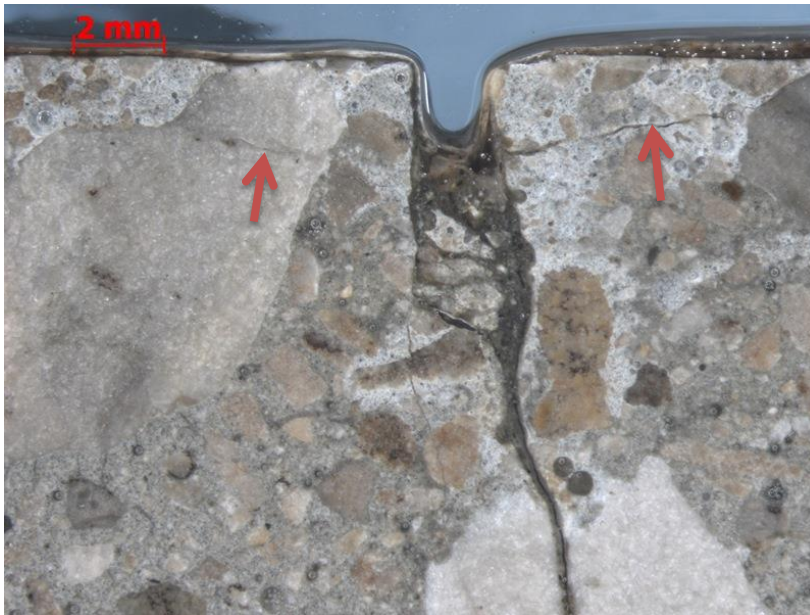
Figure 12. Core S5. Close-up view of near-top region showing a vertical crack and sub-horizontal cracks (red arrow). The vertical crack passes through a coarse aggregate particle. Epoxy was applied to the top surface to preserve the texture.
