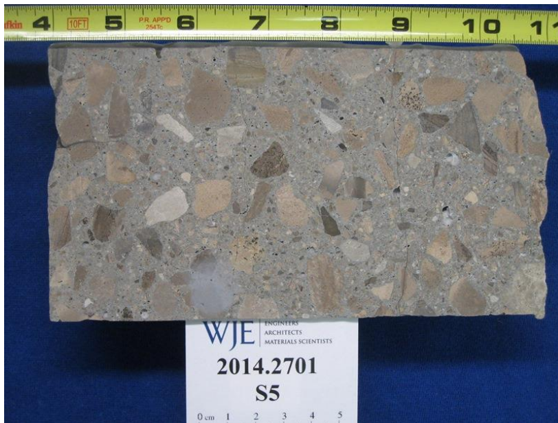
Figure 4. Core S5. Lapped cross section illustrating the appearance of the concrete. In-service top end is on left.
