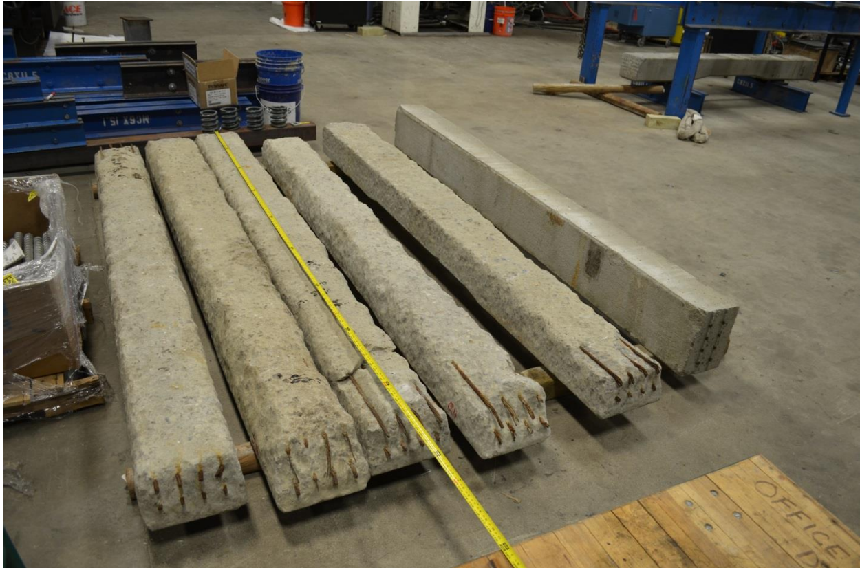
Figure 2. Overall view showing in service bottom face of railroad ties S3, N16, S4, N10 and S5, from left to right. The un-used specimen is seen seated on its side. Note the significantly abraded bottom and side surfaces of the used specimens
