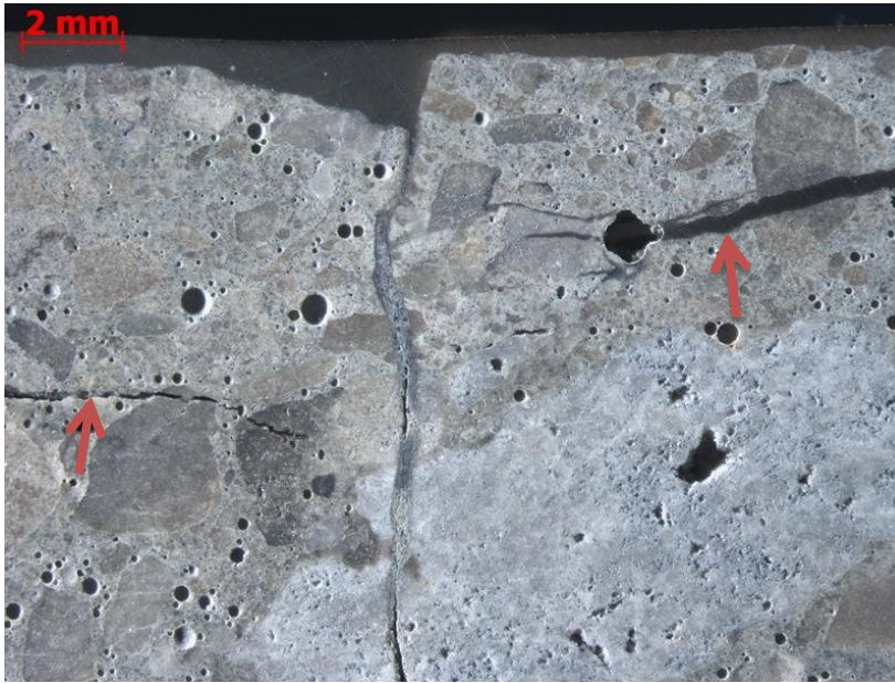
Figure 13. Core N10. Close-up view showing a vertical crack that passes through a coarse aggregate particle, and example of air-void system in the near-top region. Red arrows show discontinuous sub- horizontal cracks. Epoxy was applied to top surface to preserve the texture.
