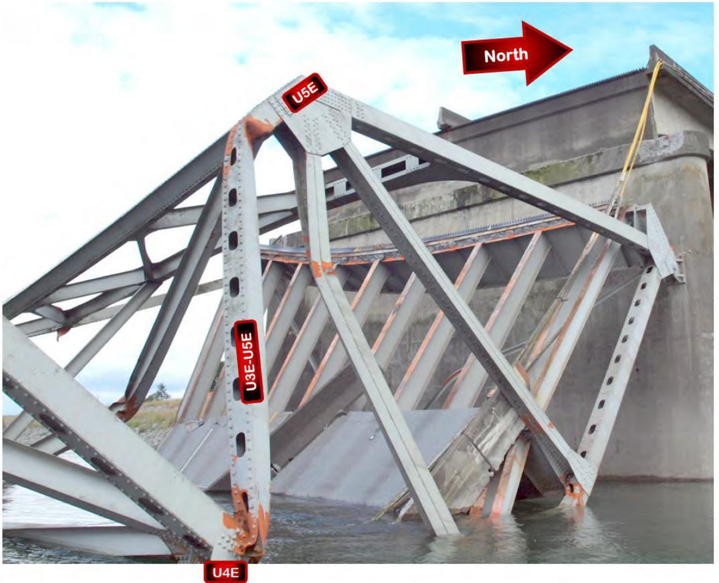
Figure 14. Nodes U5E and U4E on the collapsed structure.
