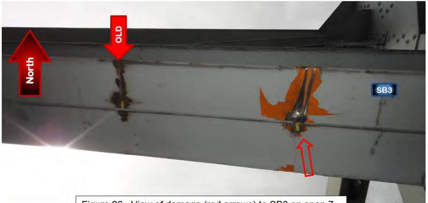
Figure 26. View of damage (red arrows) to SB3 on span 7.
