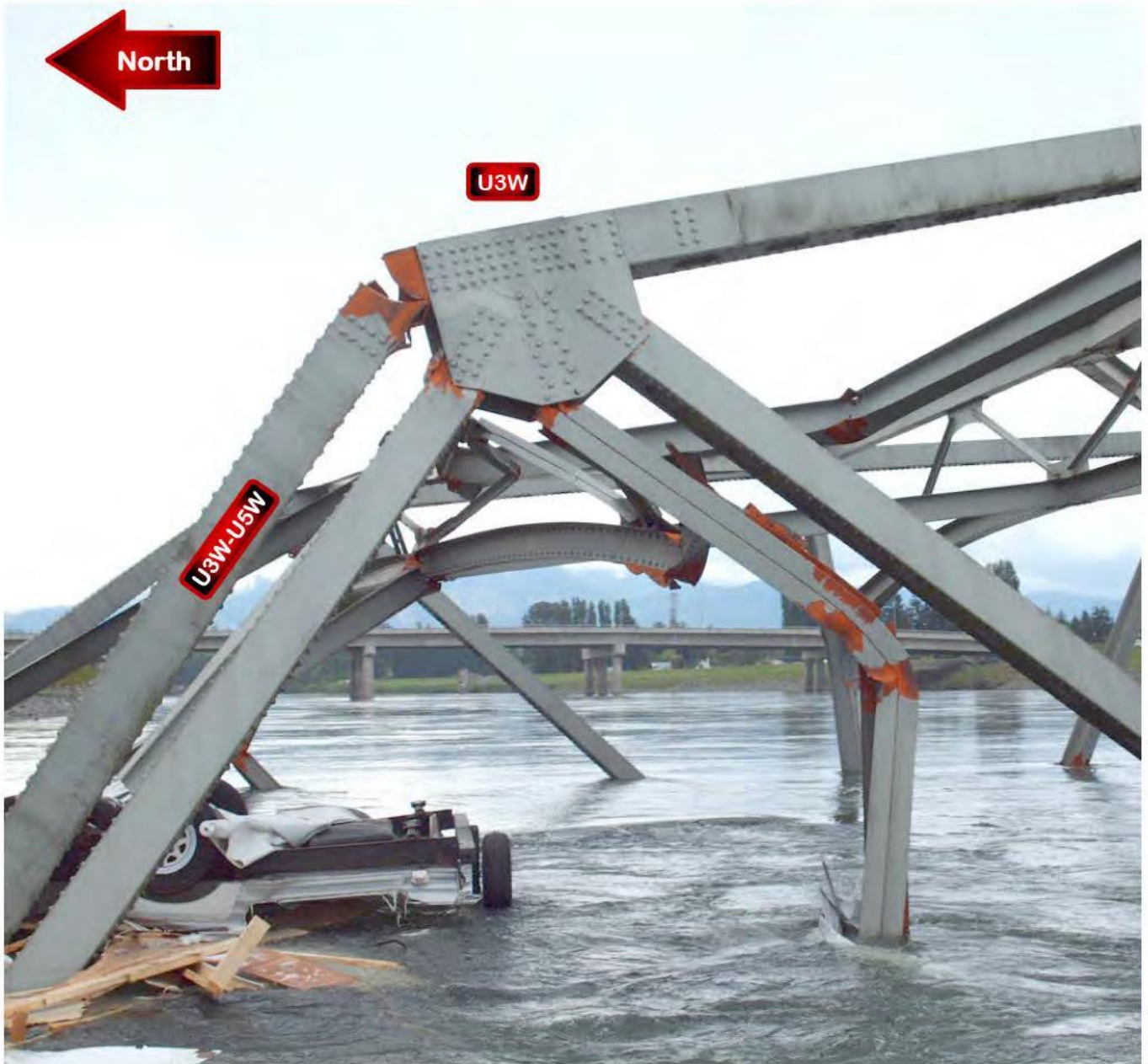
Figure 6. A view of node U3W and the surrounding damage.
