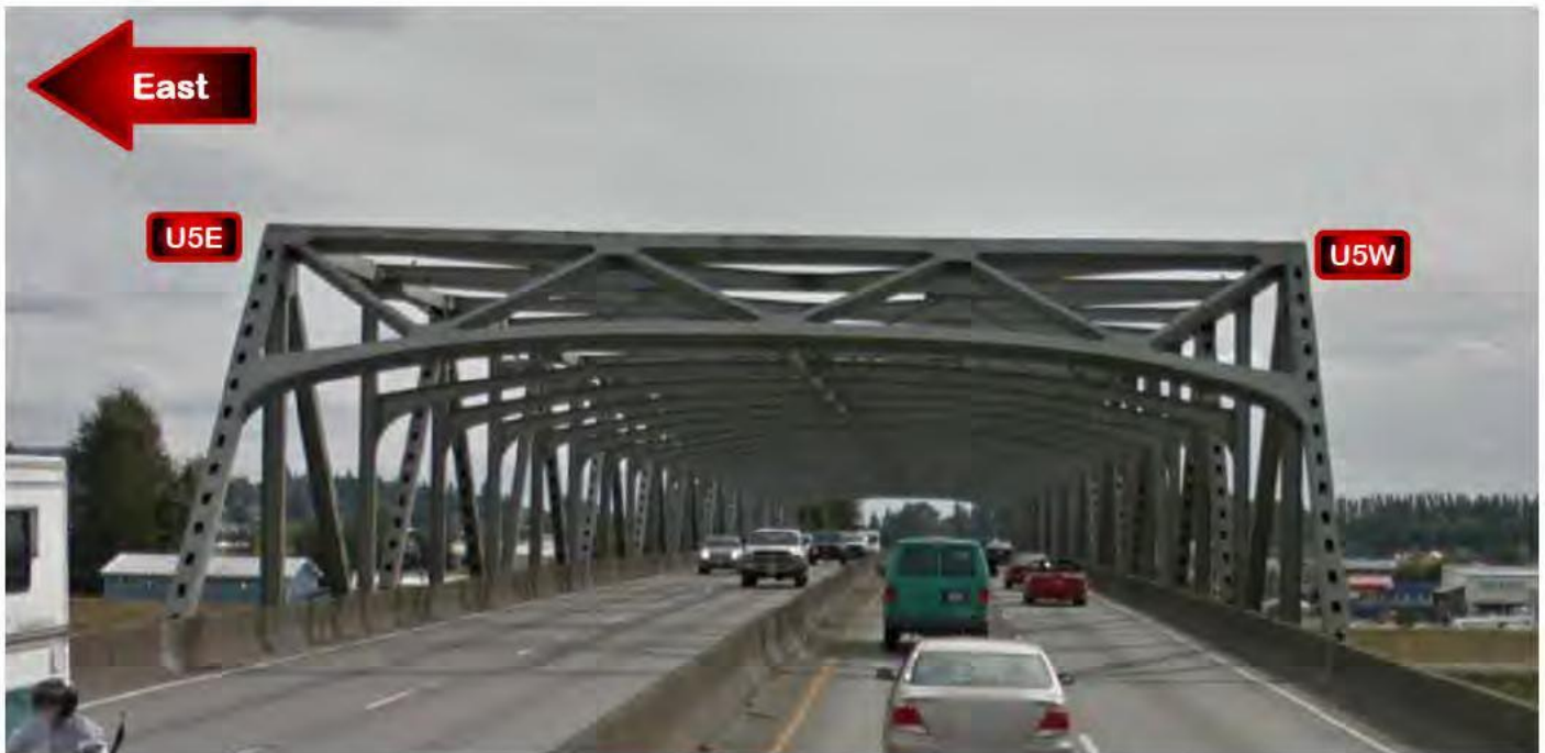
Figure 3. View looking south at the north portal prior to the collapse.
