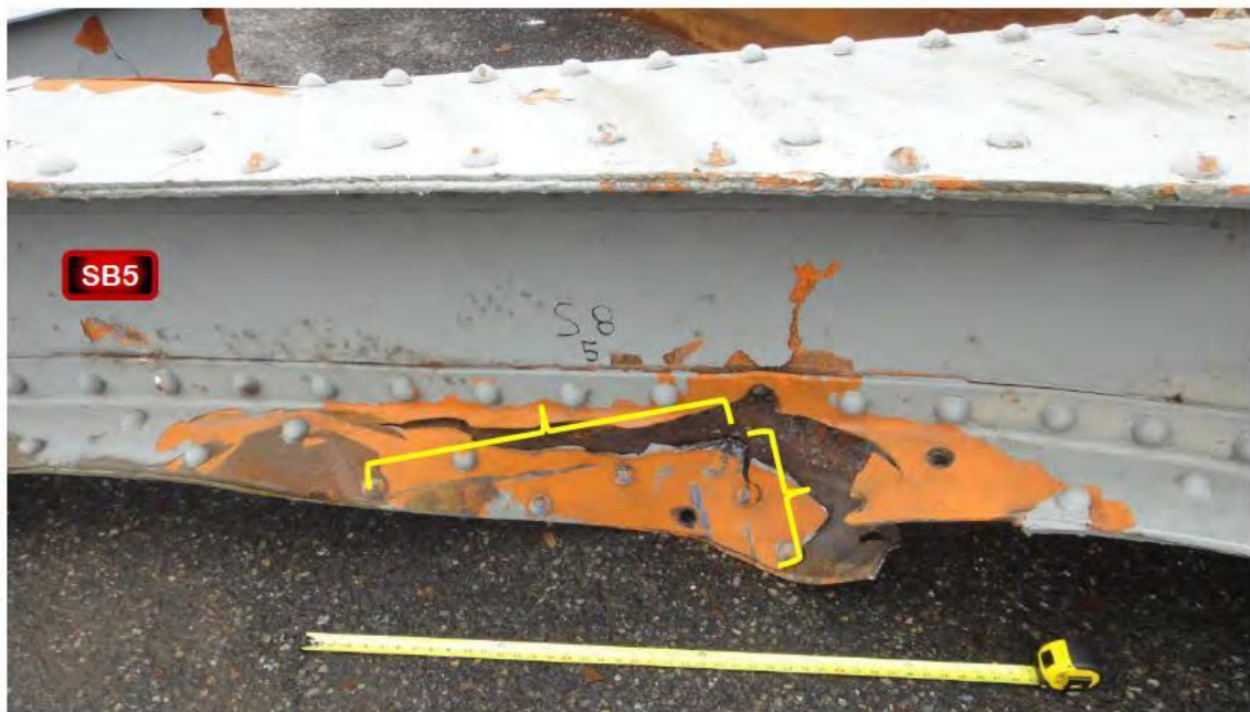
Figure 15. Impact damage to the north portal over the outside travel lane, yellow box in the upper view. A corner shape was evident in the damage as indicated by the yellow brackets in the lower view.
