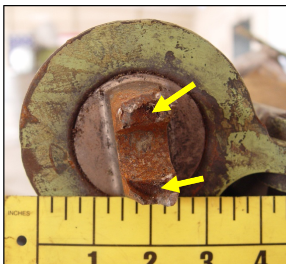
Figure 28. The outboard forward engine attachment indicated by the green arrow in Figure 27 and in Figure 5.
