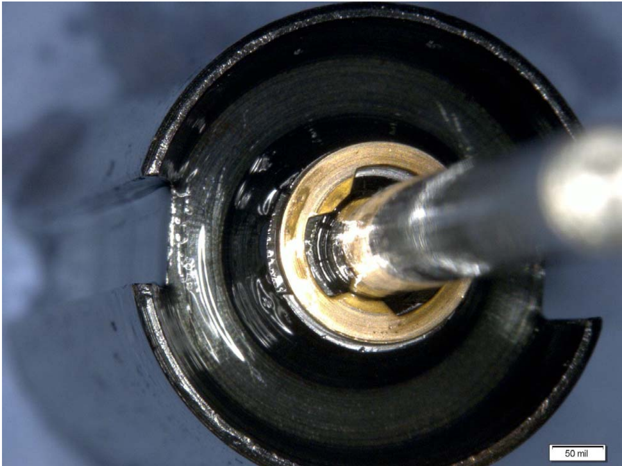
Figure 15: The steering control valve number 5 armature, with a bronze ring of different design than that found in the propulsion control valve.
