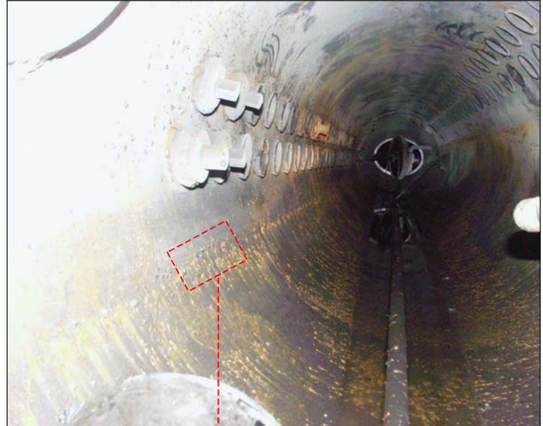
HEADER FROM BOILER #21
