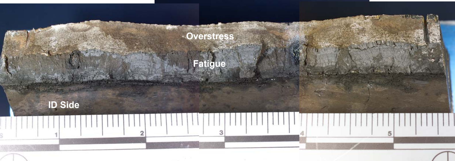
Figure 28: Views of the tube sheet fracture on Section 6 taken from the upper longitudinal weld of header 23. The upper image is a view of the fracture surface and ID surface at an angle, while the lower image is a more straight-on view of the fracture surface.
