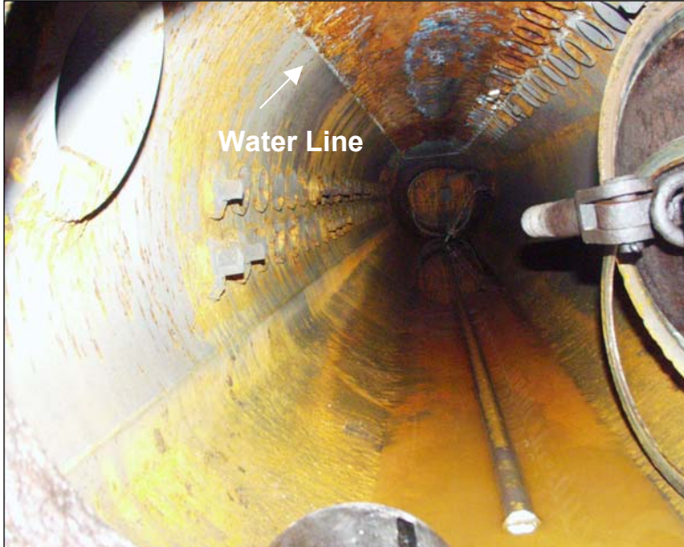
HEADER FROM BOILER #24
