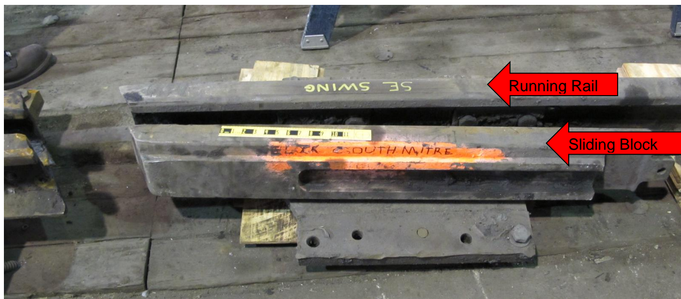
Figure 8. View of the south side east rail lock showing extensive damage to the bridge side components including; separation of the guide rail section with fracturing of the attaching bolts and release of the sliding block. View looking west.
