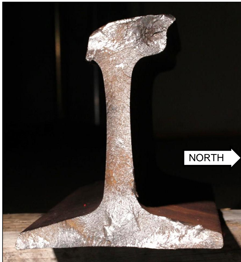
Figure 5. Views of the fracture surface at the east end of piece N5. A dashed line in the closer view of the head indicates the boundary of a detail fracture emanating from the gage corner.
