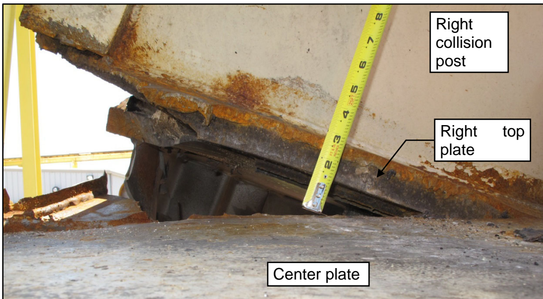
Figure 3. Side view of the lower end of the right collision post looking outward.
