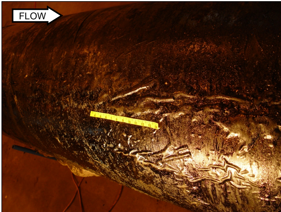
Figure 5. 3 o'clock position on the pipe piece B showing wrinkles in the coating.
