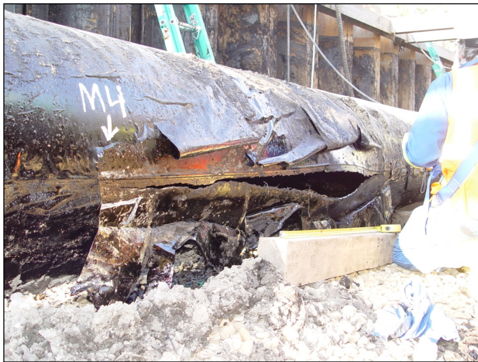
Figure 2. Views of the pipe in the trench showing the rupture location.
