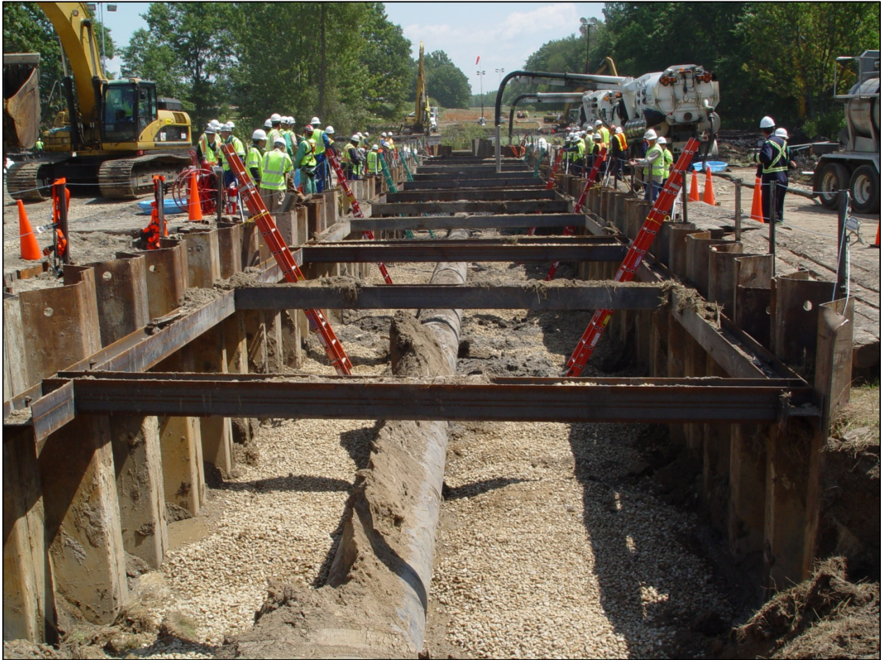
Figure 1. Overall view of the pipeline within the trench dug at the accident scene as viewed facing east.
