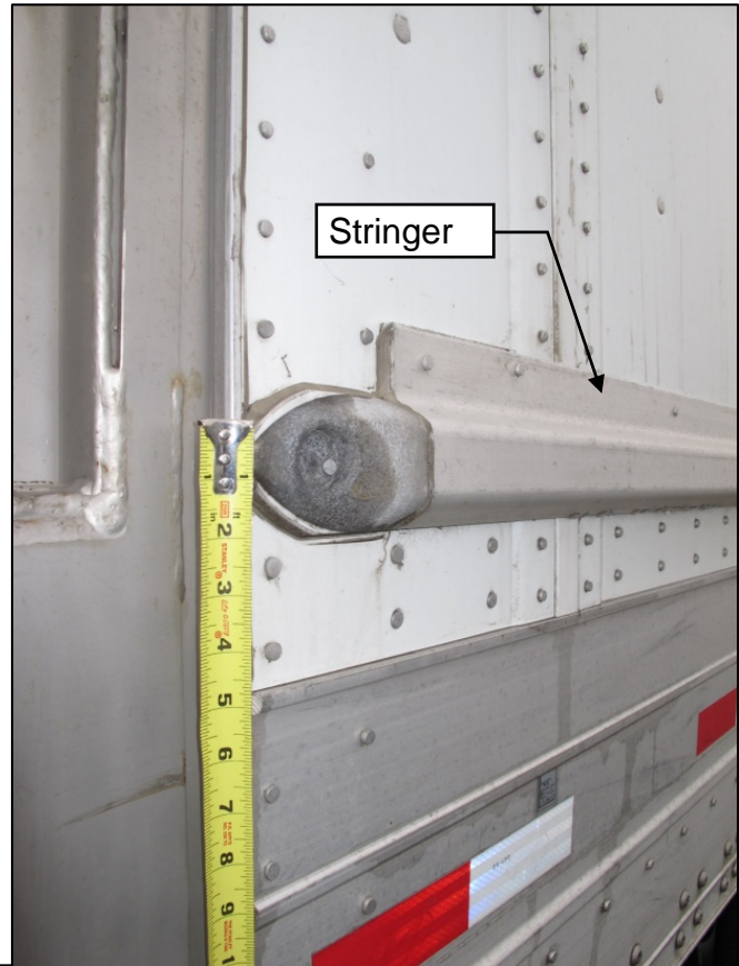
Figure 8. Oblique view of the rear end of the lower stringer on the right side of the trailer.
