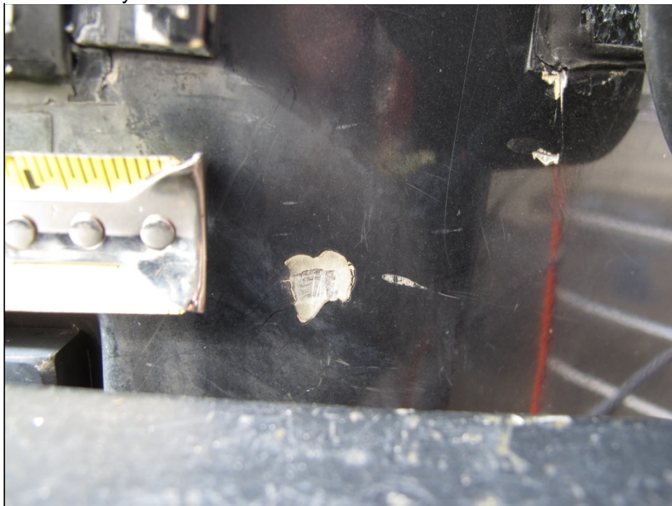
Figure 17. Closer view of contact damage labeled B in figure 16.
