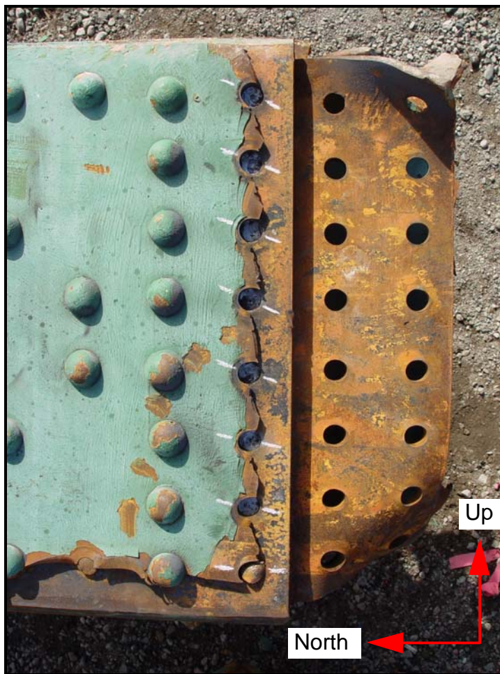
Figure 24. View of the deformation pattern associated with the fracture in the west gusset plate at node U10' East in the area of the upper chord (after grinding off the heads of the rivets adjacent to the fracture). Markings that indicate the tensile loading direction have been added through the rivet holes adjacent to the fracture. Compare to the left photograph in figure 15.
