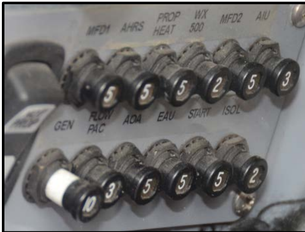
Figure 27: Generator Circuit Breaker
