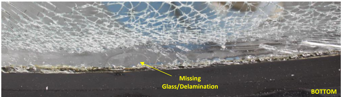
Figure D: Close-up View of Delamination
