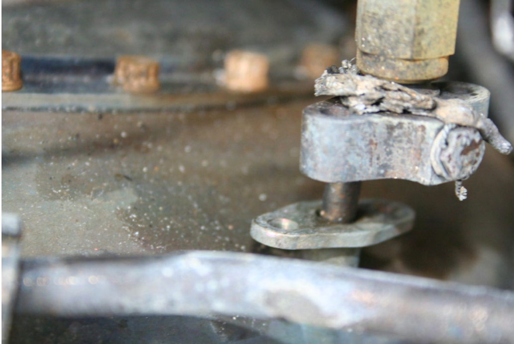
Photo 2. Fuel Inlet Union at Attach Point
