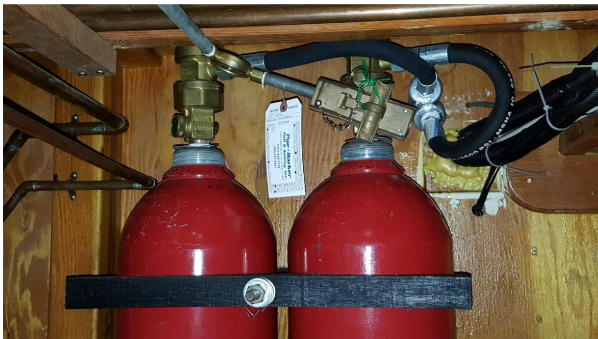
Figure 18. Components of the Island Lady 's fixed fire suppression system in March 2017 before the fire. (Photo by the Coast Guard)
