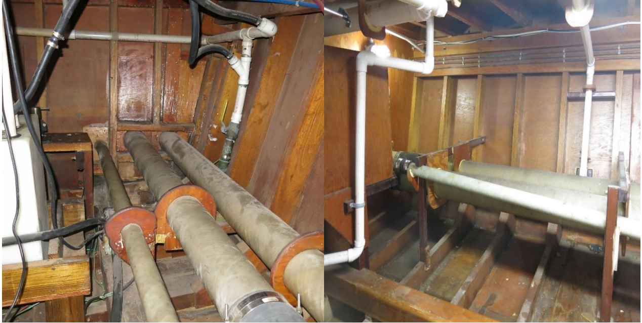
Figure 15. Engine exhaust tubes transiting through the lazarette spaces on board vessels constructed similarly to the Island Lady .
