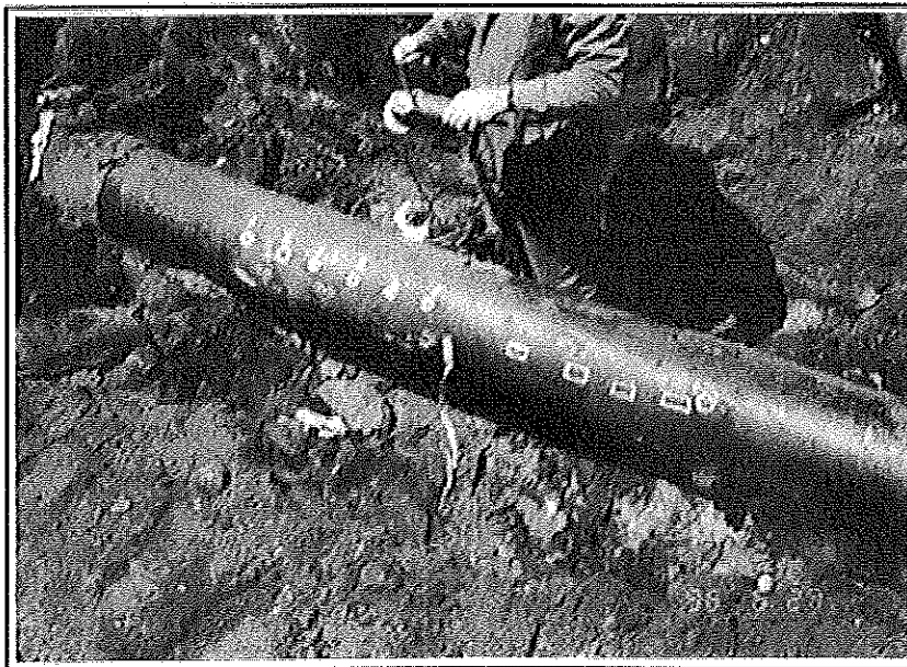
Figure 2 (bottom). Pipe during inspection. White round circles indicate leaks. Note their linear arrangement along the longitudinal axis of the pipe.
