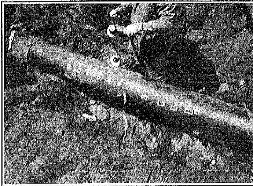
Figure 2 (bottom). Pipe during inspection. White round circles indicate leaks. Note their linear arrangement along the longitudinal axis of the pipe.
