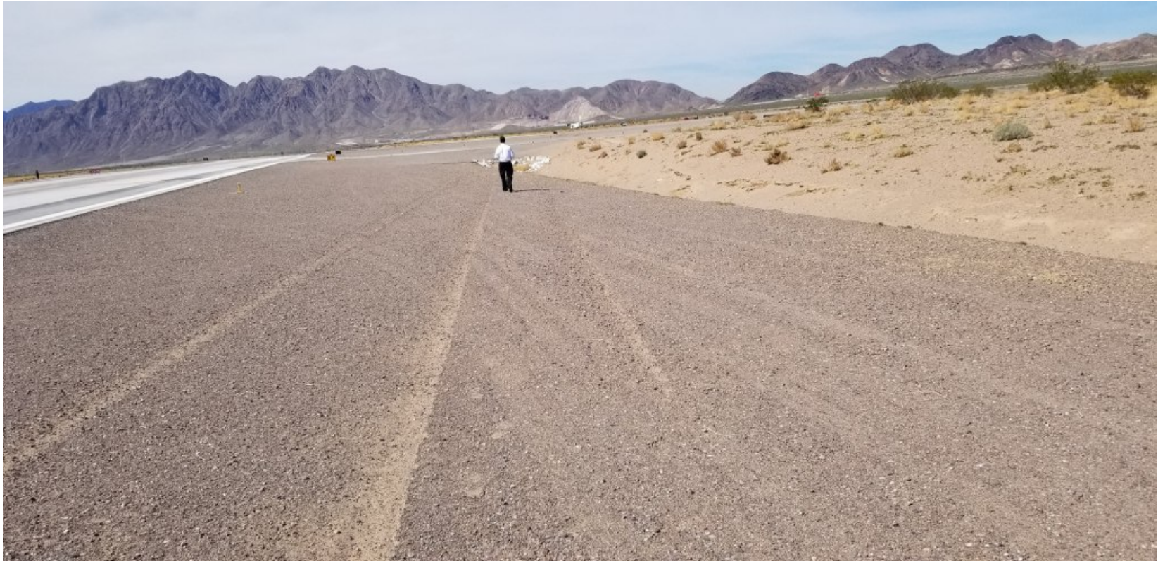
Figure 3 - Tire Track Marks and Ditch
