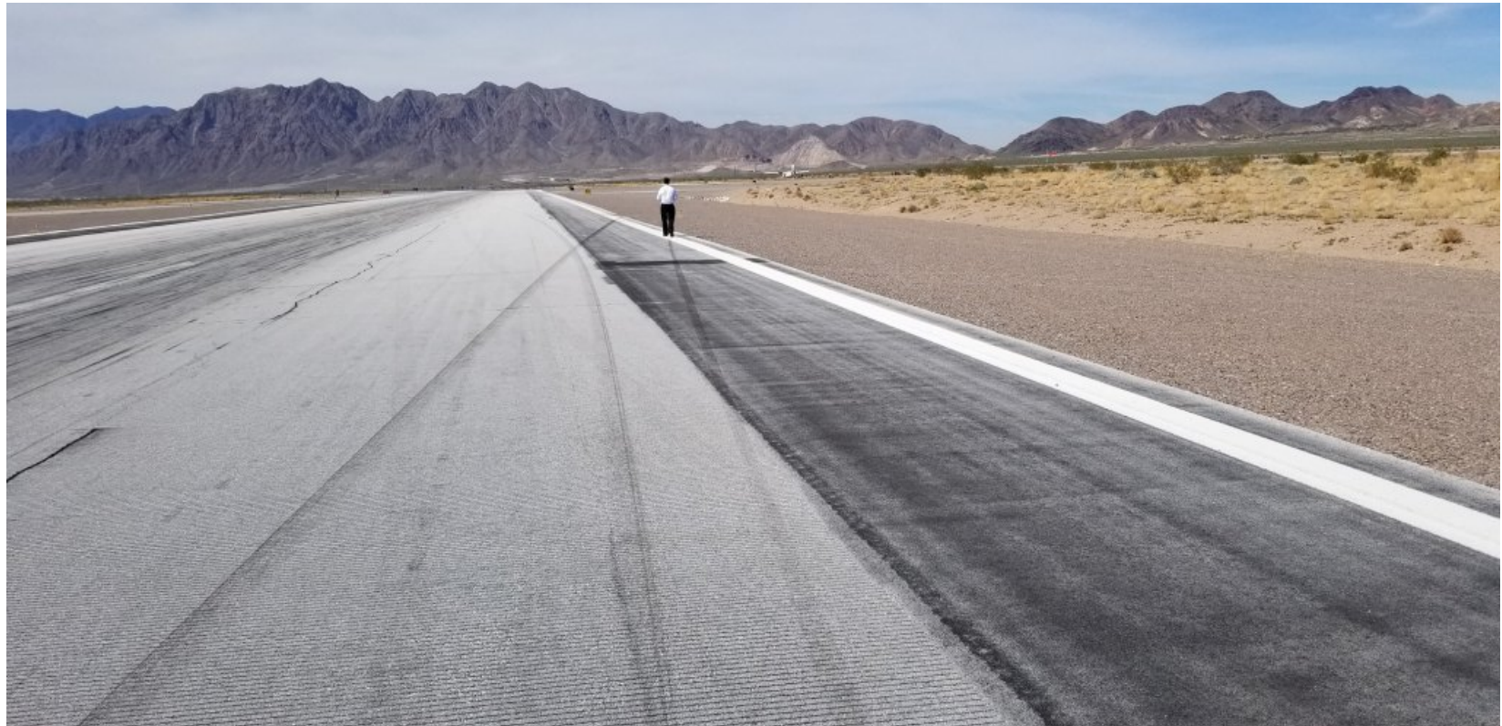
Figure 1 - Tire Track Marks Exiting Runway
