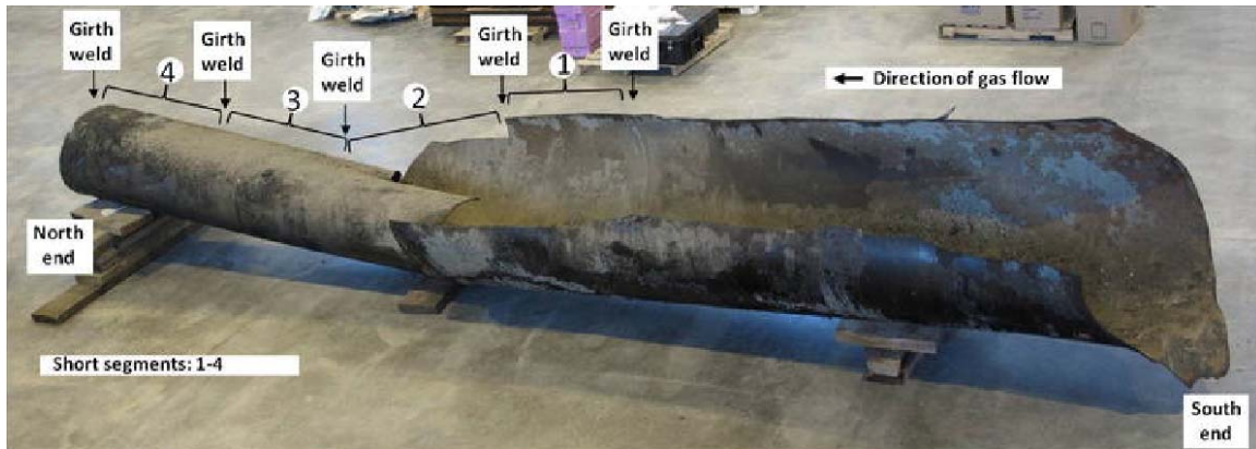
Figure 6 - Photograph of 28-foot-long ruptured section of pipeline Segment 180 40
