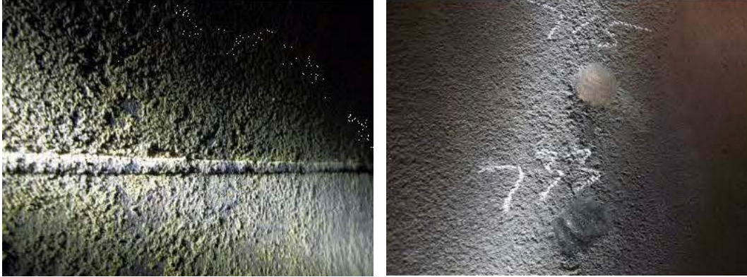
Figure 6: AXLX1702 internal corrosion and ultrasonic thickness measurement locations in Ring 2, Rescar inspection March 21, 2016.
