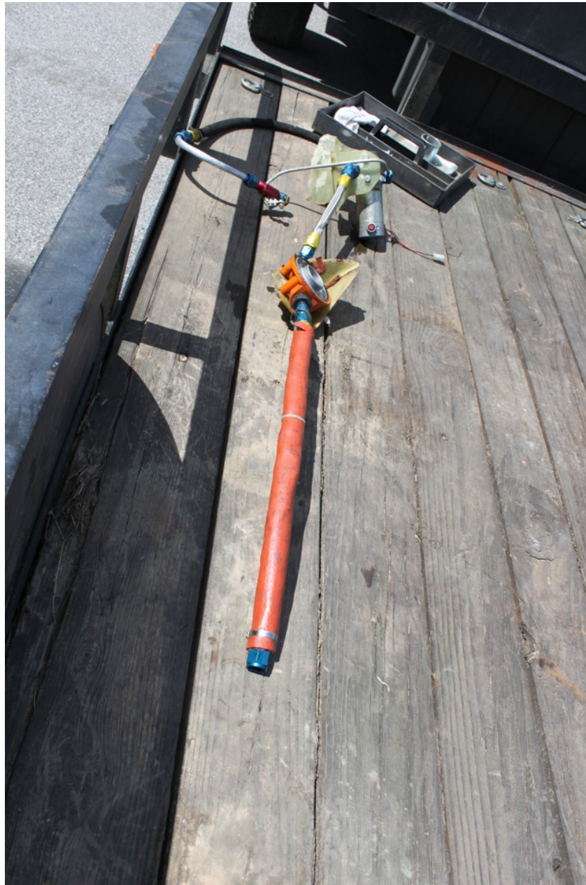
Photo 10 - NTSB Digital Photograph. View of the Fuel Supply System Including Lines from the Fractured Fuel Tank Outlet Fitting, Shutoff Valve, Auxiliary Fuel Pump, Fuel Filter, and Fuel Line to Engine-Driven Fuel Pump.
