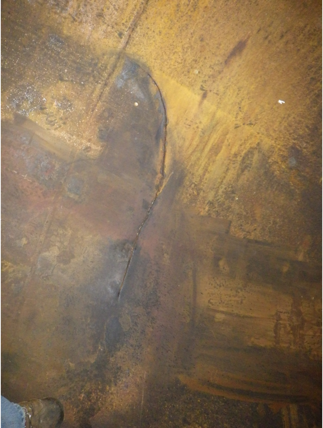
Interior tank shell view showing length of the crack in Ring 4, August 31, 2016
