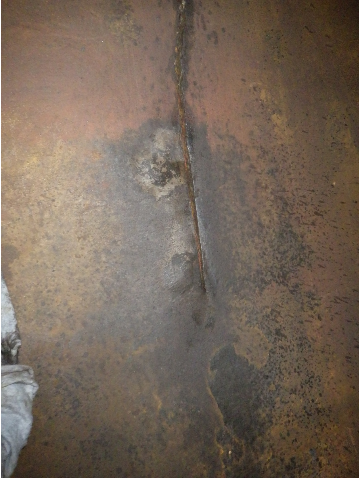
Interior corrosion repair spots inboard of cradle pad termination adjacent to shell crack, August 31, 2016.
