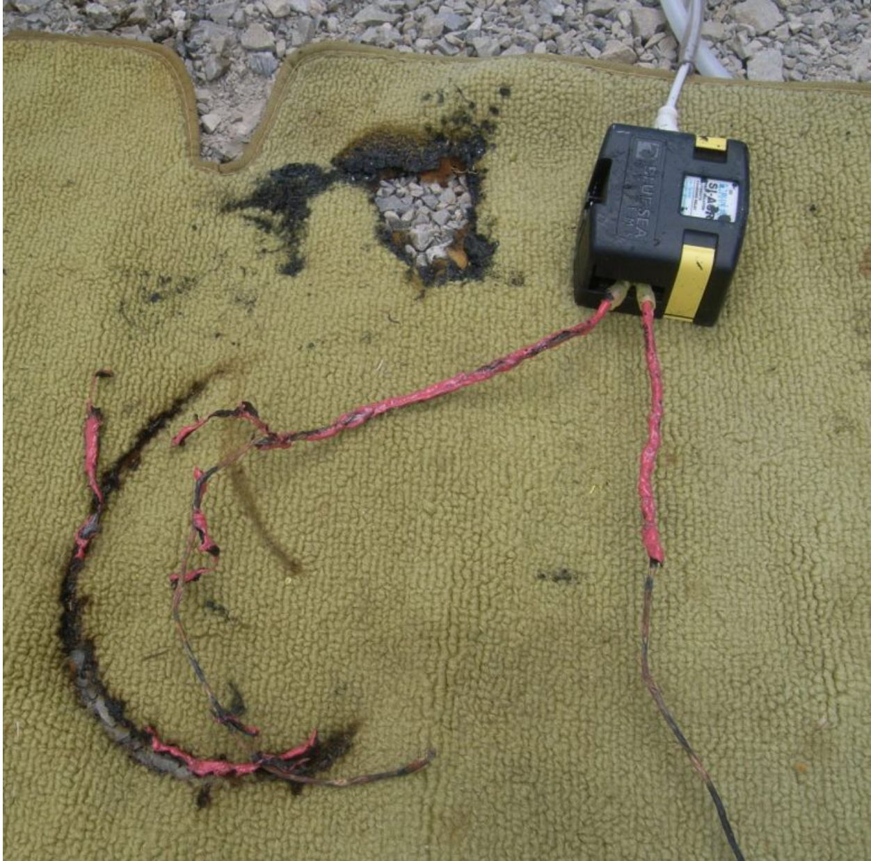
Figure 47 - Burned Isolator, Wires, and Carpet
