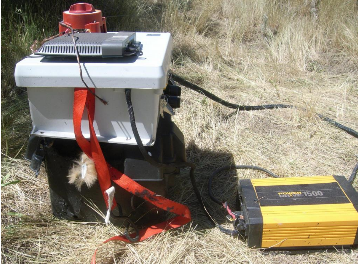
Figure 37 - Stackup of Battery, Distribution Box, and Modem & Switch (view from airplane right)
