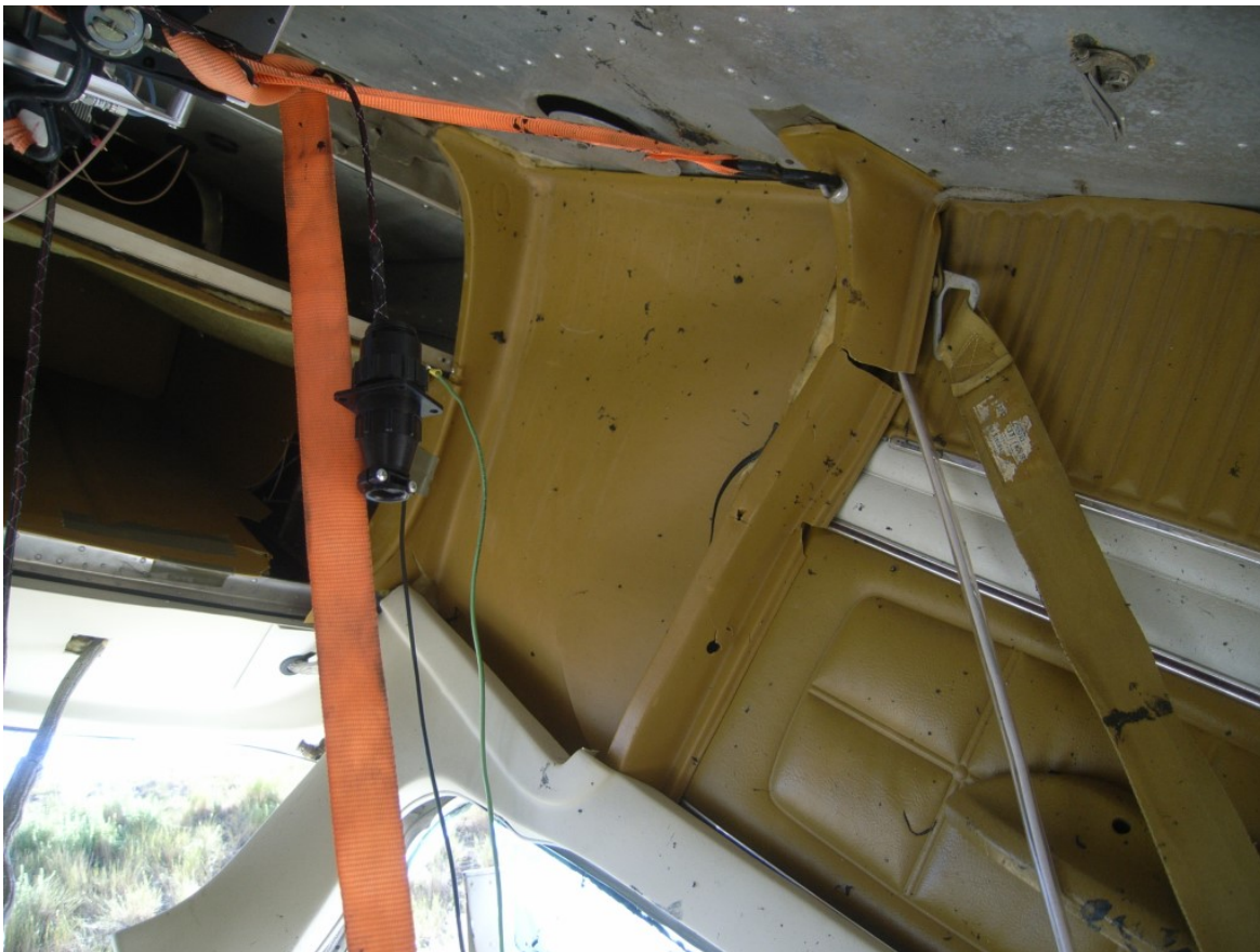
Figure 32 - Cabin Sidewall with Melted Deposits
