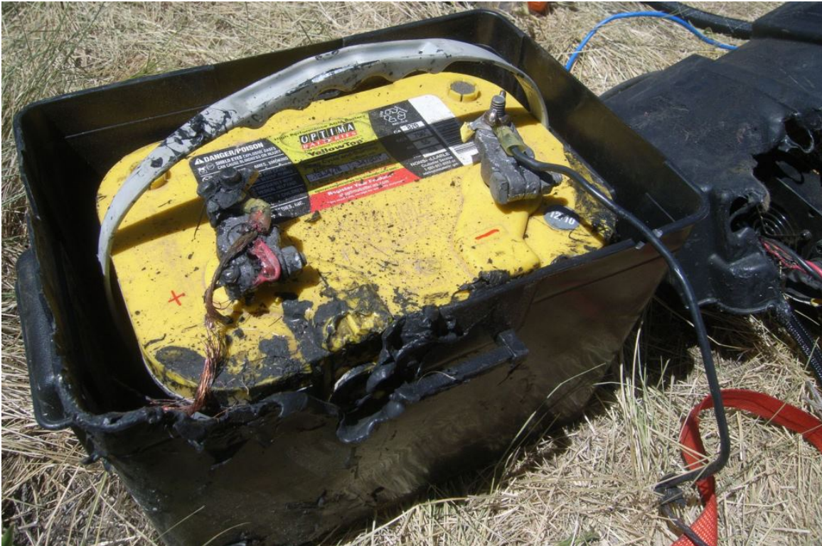
Figure 41 - Battery in Battery Box
