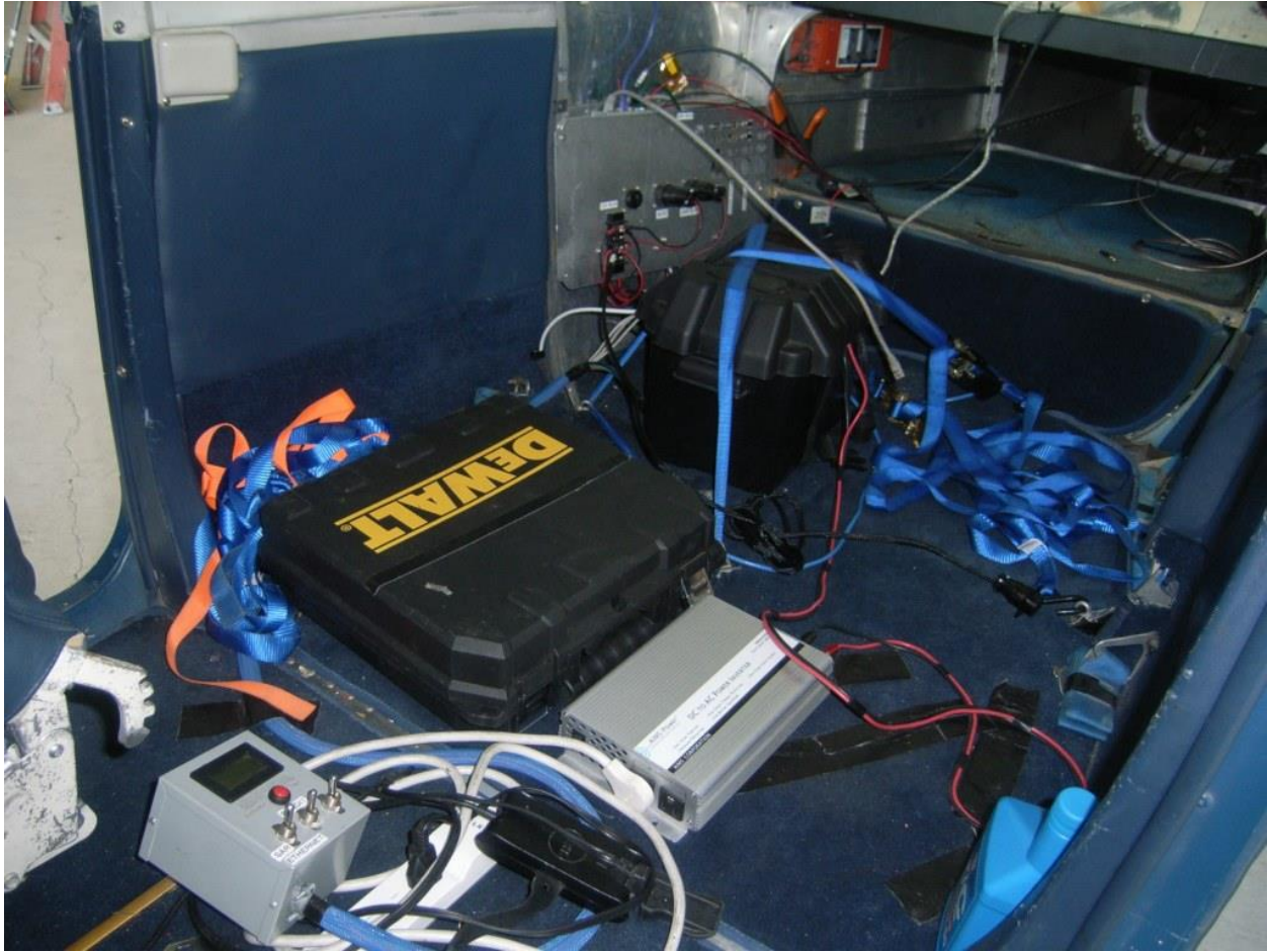
Figure 48 - Supplemental Power Supply (undergoing revision)
