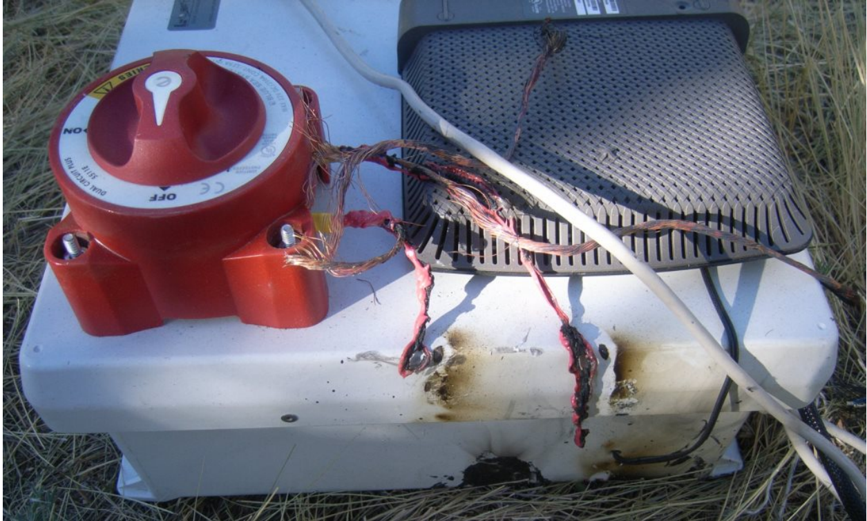
Figure 44 - Battery Switch & Modem on Distribution Box
