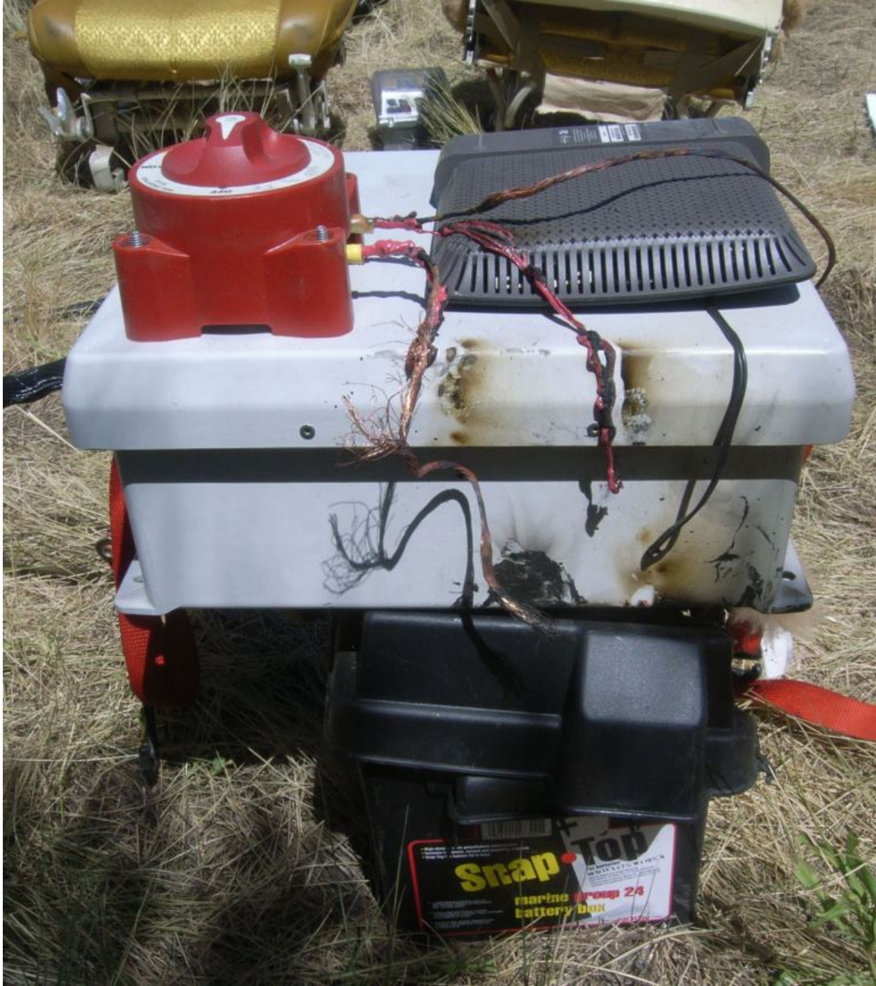
Figure 38 - Stackup of Battery, Distribution Box, and Modem & Switch (view forward)
