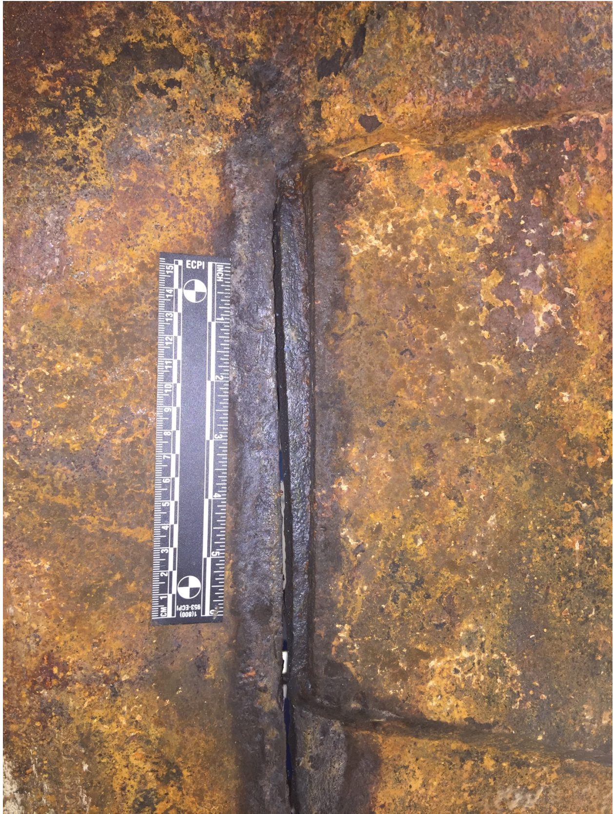
Inboard end of A-End cradle pad and tank crack
