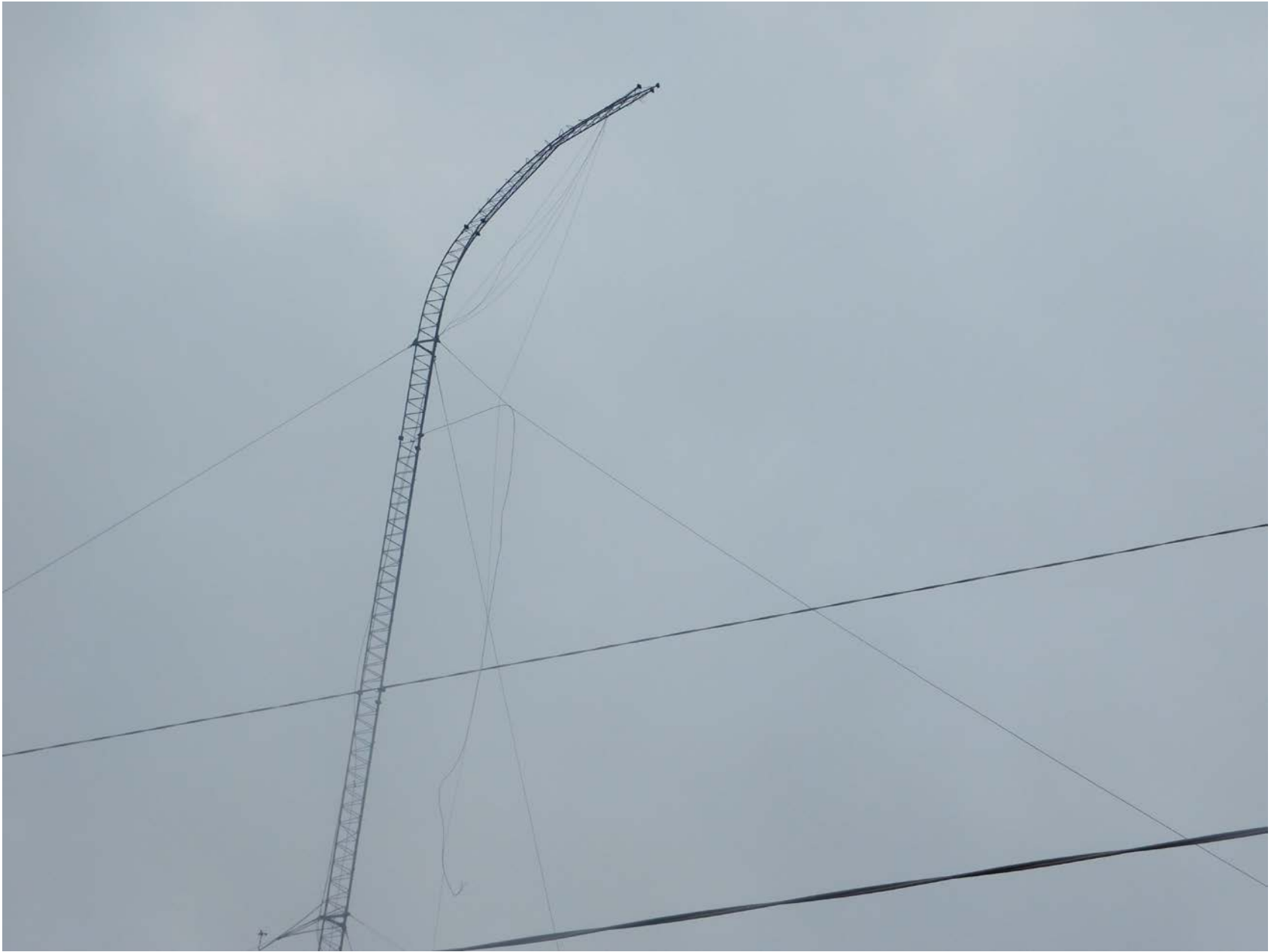
Photo 1 – View of tower damage
