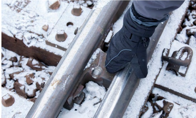
2 3 Figure 35. Strike mark located at left hand switch point heel block
