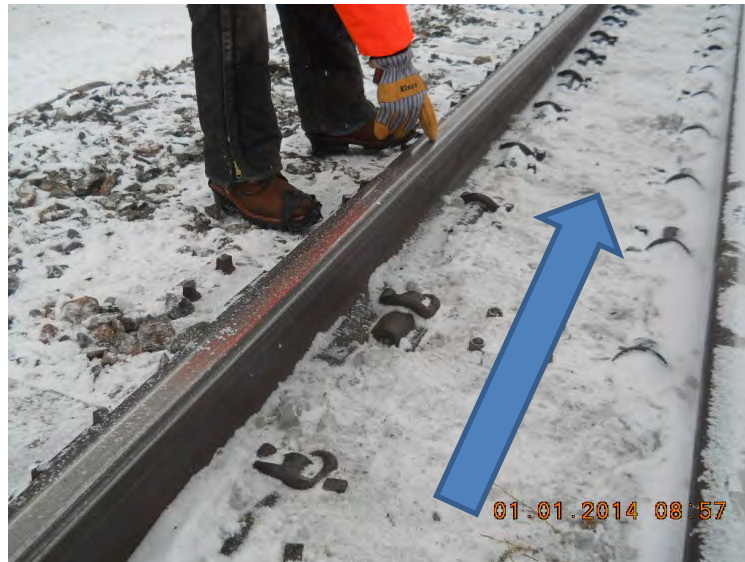
31 Figure 14. View of derailment marks; blue arrow indicates direction of train travel. 32 33 34 35 36 37 38 39 40
