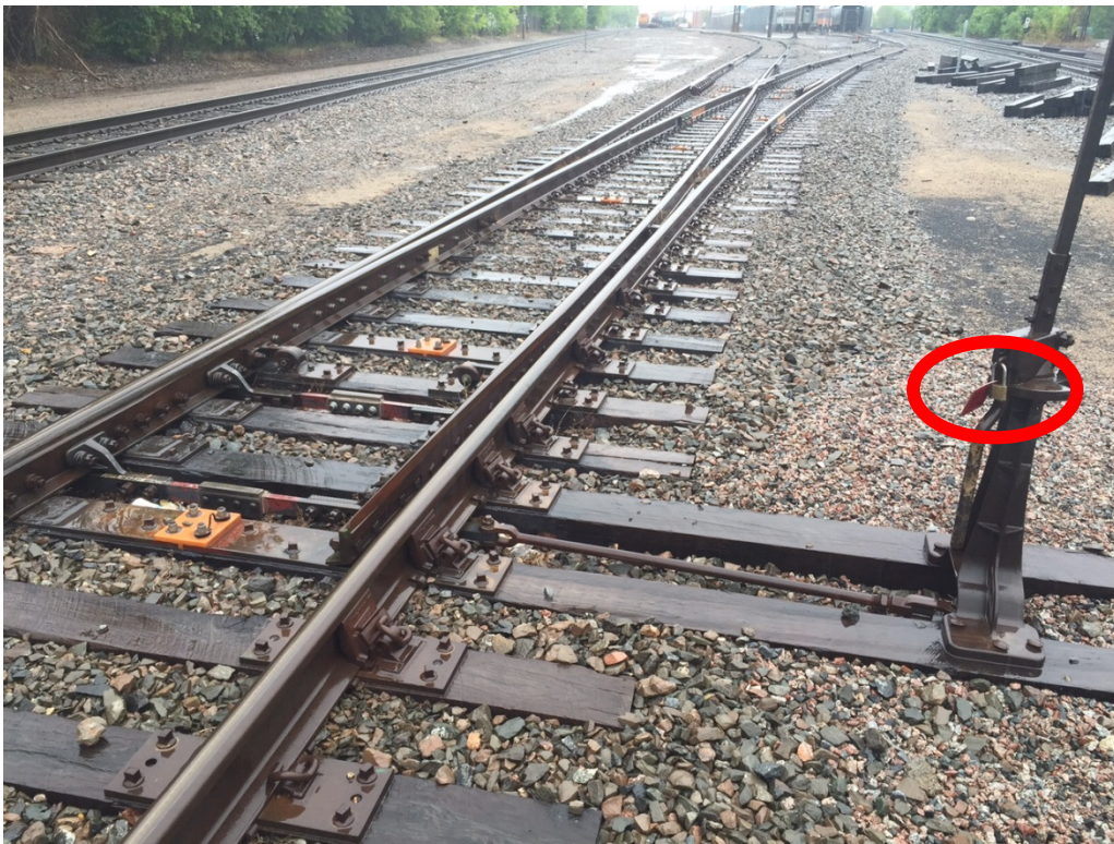
Figure 2. A view of the west switch leading into the Old Main 2 Pocket track lined toward another track. The red circle shows where a maintenance of way lock had been applied.
