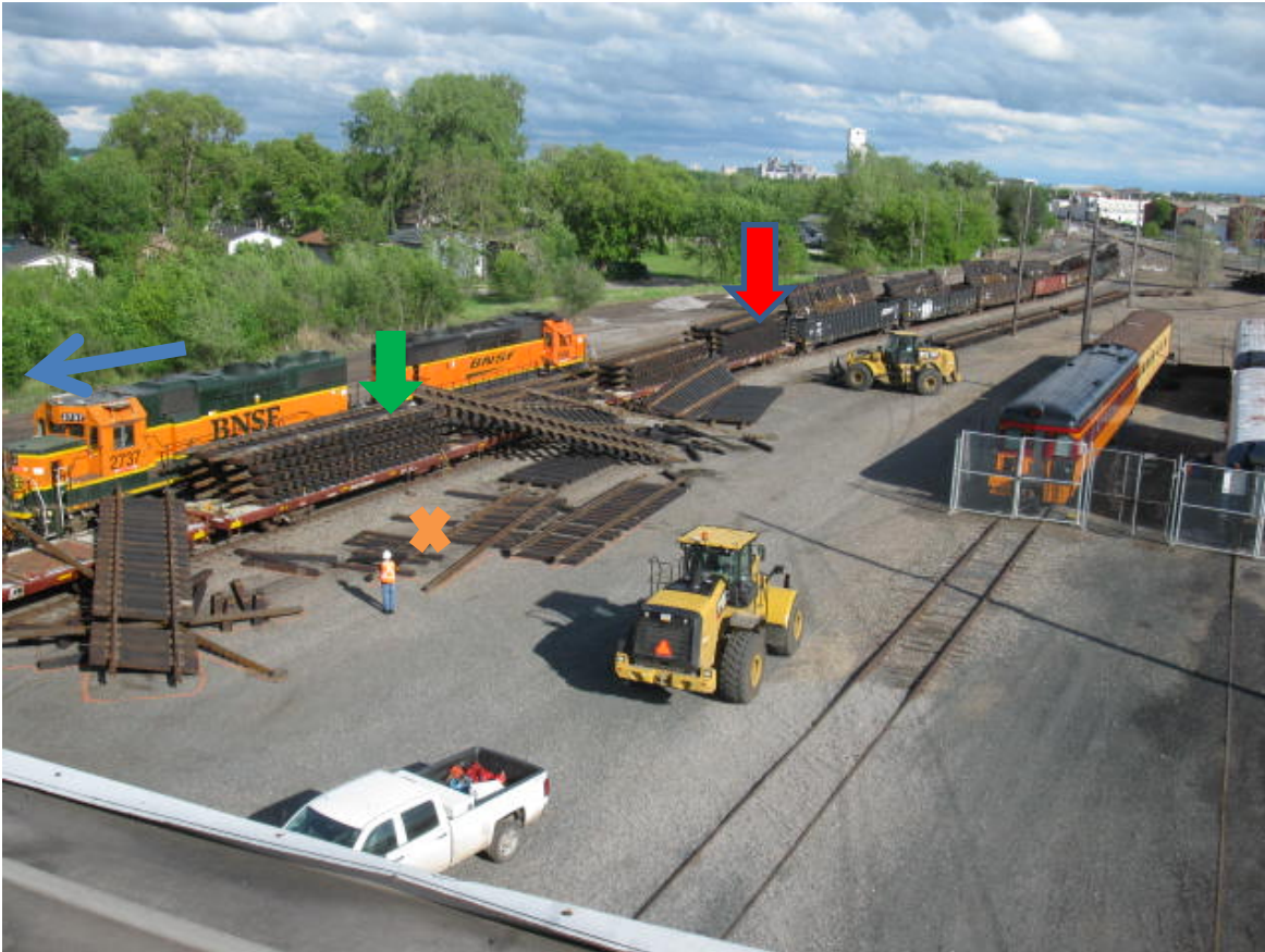
Figure 1. This is a view looking southeast at accident scene where loader in the background had attempted to lift two track panels (see red arrow). There are two loaded flat cars with two stacks of track panels per car, seven track panels to a stack. Blue arrow indicates direction of travel of locomotives. Green arrow points to likely position of foreman atop a stack of track panels as indicated by train crew. Orange “x” is approximate location of deceased.
