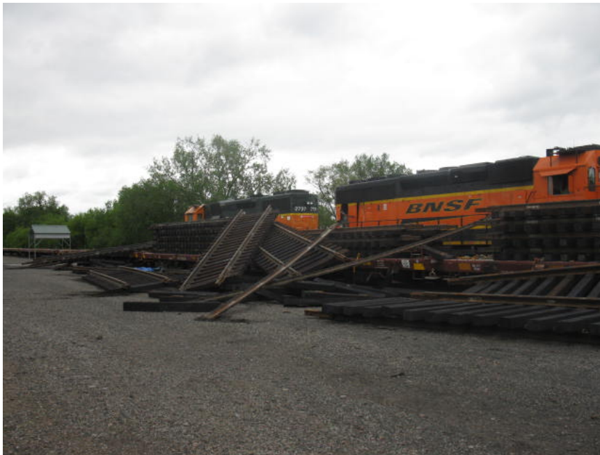
Figure 7. This is a view of dislodged track panels.
