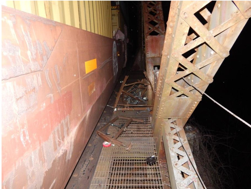
Figure 3. Walkway on the east side of the trestle and the remnants of the bed after being struck by the train. (Photo by CSX).
