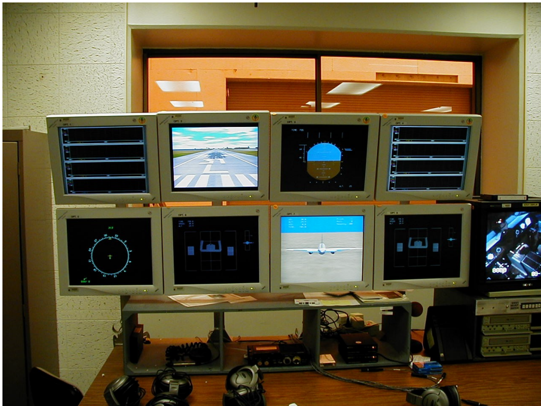
Figure 5. Control room layout.
