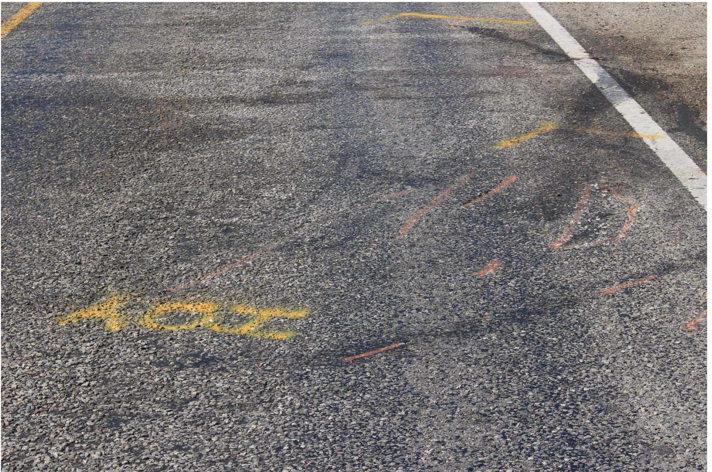
Highway Photo 37 – Southbound view of the impact area in the southbound lane.
