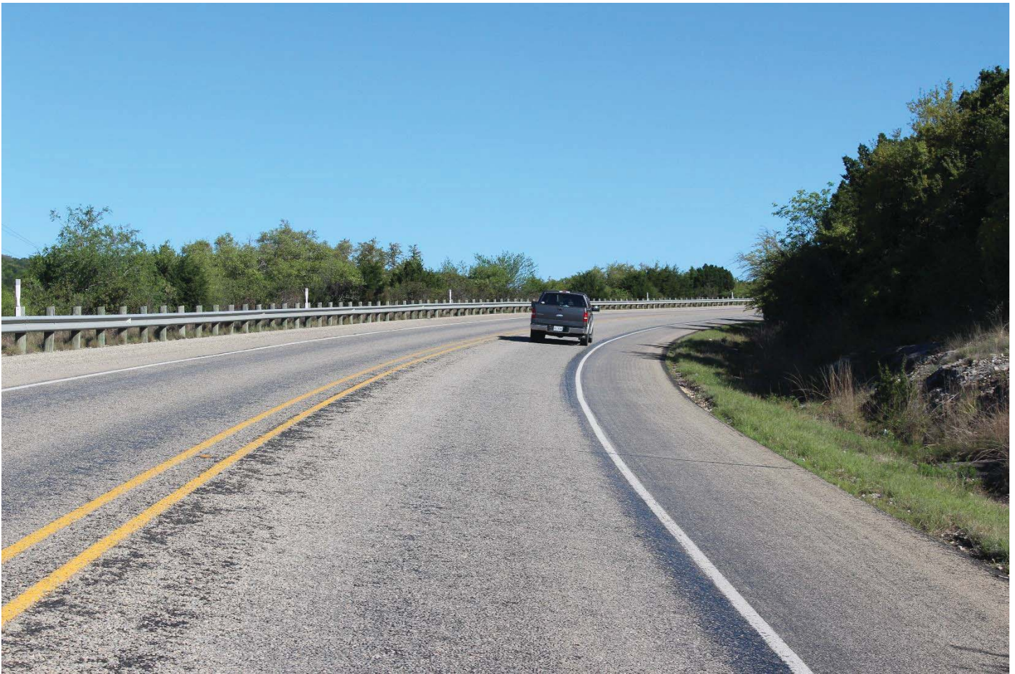
Highway Photo 17 – Note how the forward sight distance in the curve is limited by the cut slope and vegetation on the hill side.
