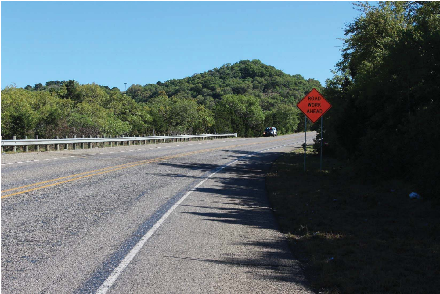
Highway Photo 28 – Northbound view of impact area in the southbound lane.
