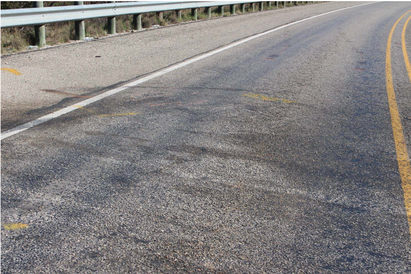
Highway Photo 31 – Close-up view of impact area in the southbound lane of US 83.
