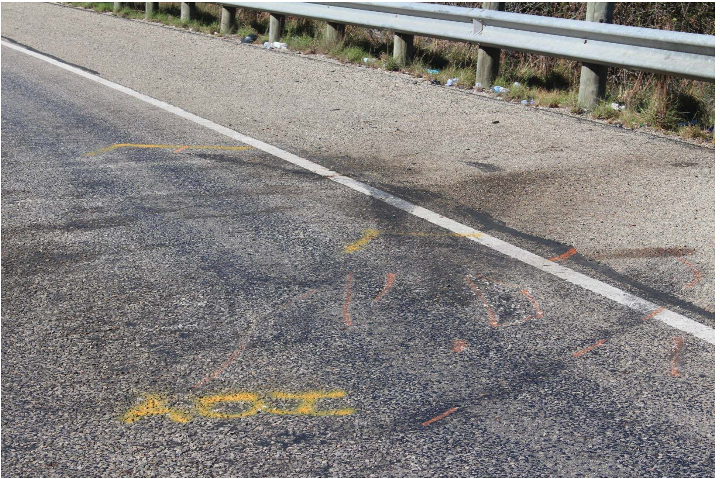
Highway Photo 38 – Additional close-up view of pavement gouges and tire friction marks in the impact area.
