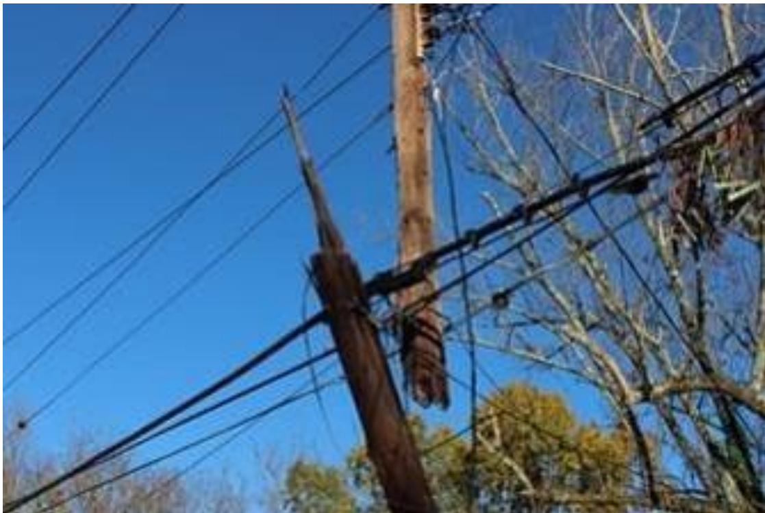
Highway Photograph 11 – View of the damaged utility pole after the crash
