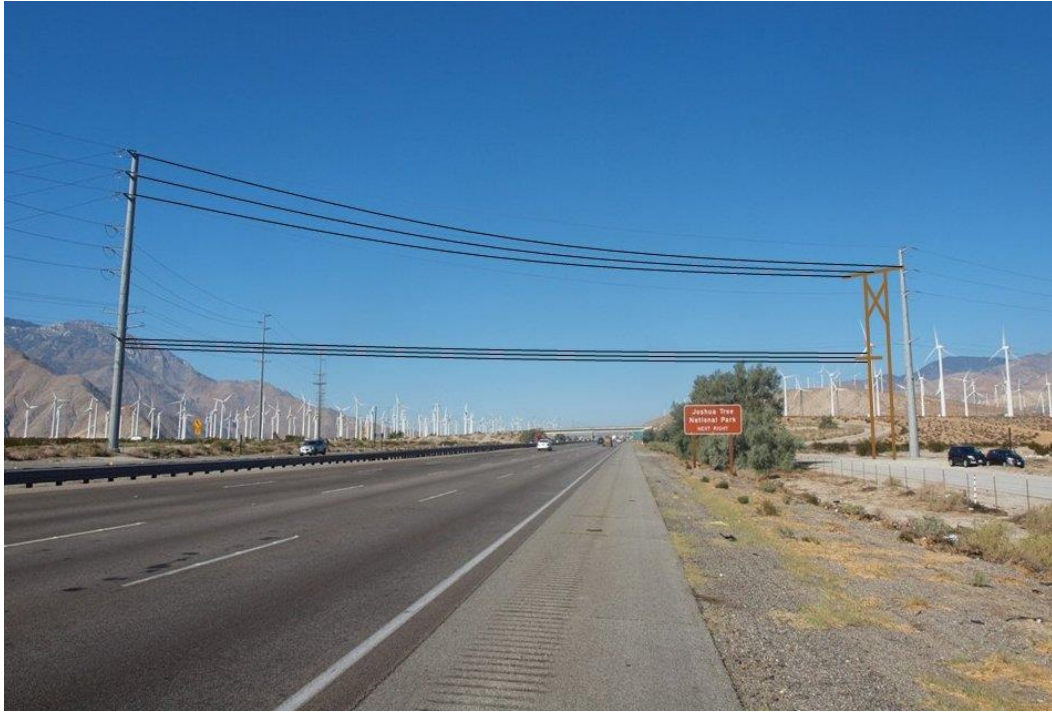
Highway Photograph 3 – Illustration depicting Stage 1 utility work. At the beginning of the utility work, the new tubular steel pole structure has no transmission lines attached to it spanning I-10. The wood structure and new steel pole structure are located side by side.
