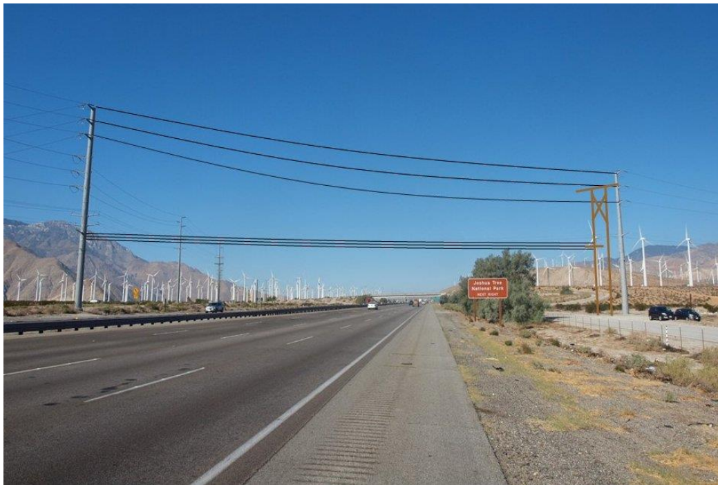
Highway Photograph 4 – Illustration depicting Stage 2 utility work. The top 3 lines are fastened to the new steel pole structure.
