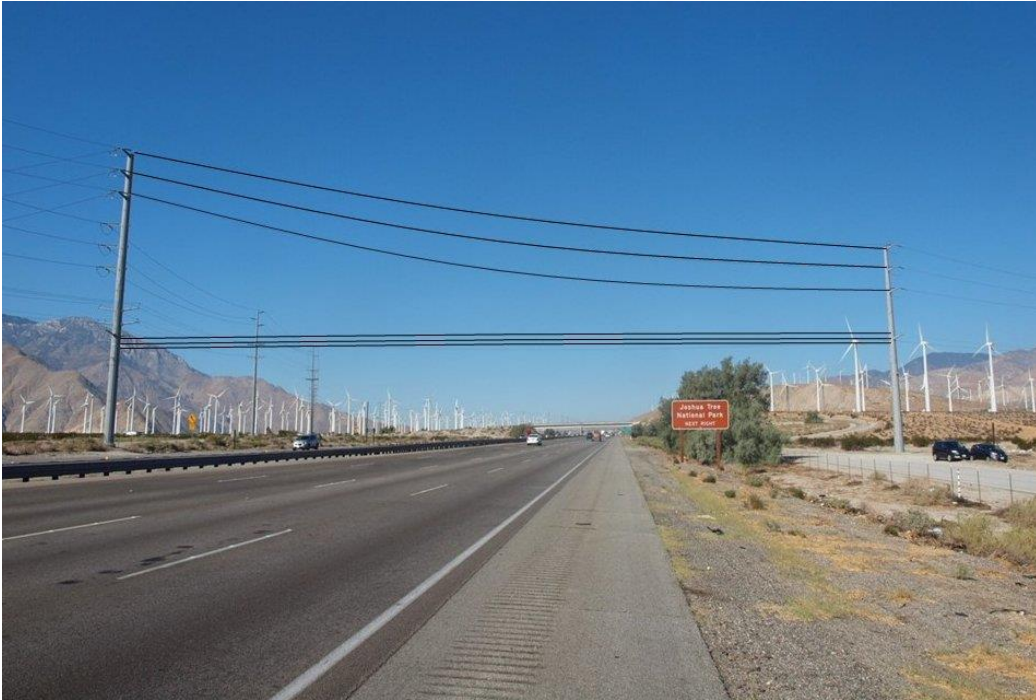
Highway Photograph 6 – Illustration depicting Stage 4 utility work. The existing H-frame wood structure is removed from the jobsite.
