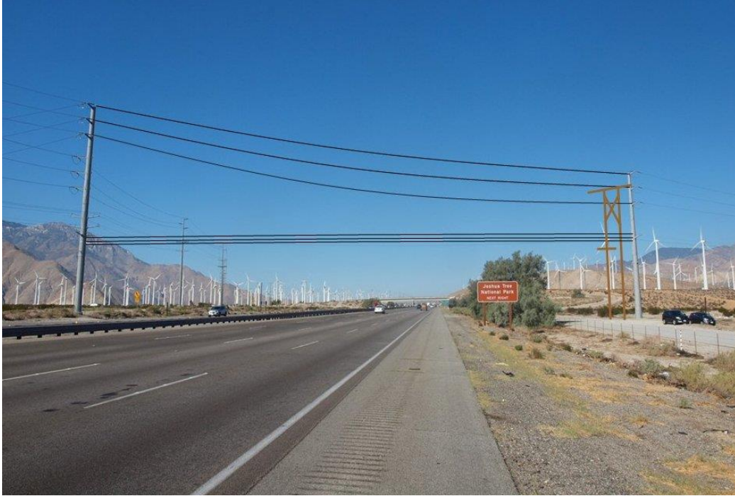
Highway Photograph 5 – Illustration depicting Stage 3 utility work. The bottom 3 lines are transferred to the new tubular steel pole. Safety devices are attached to the bottom 3 lines as an additional measure to secure the transfer.
