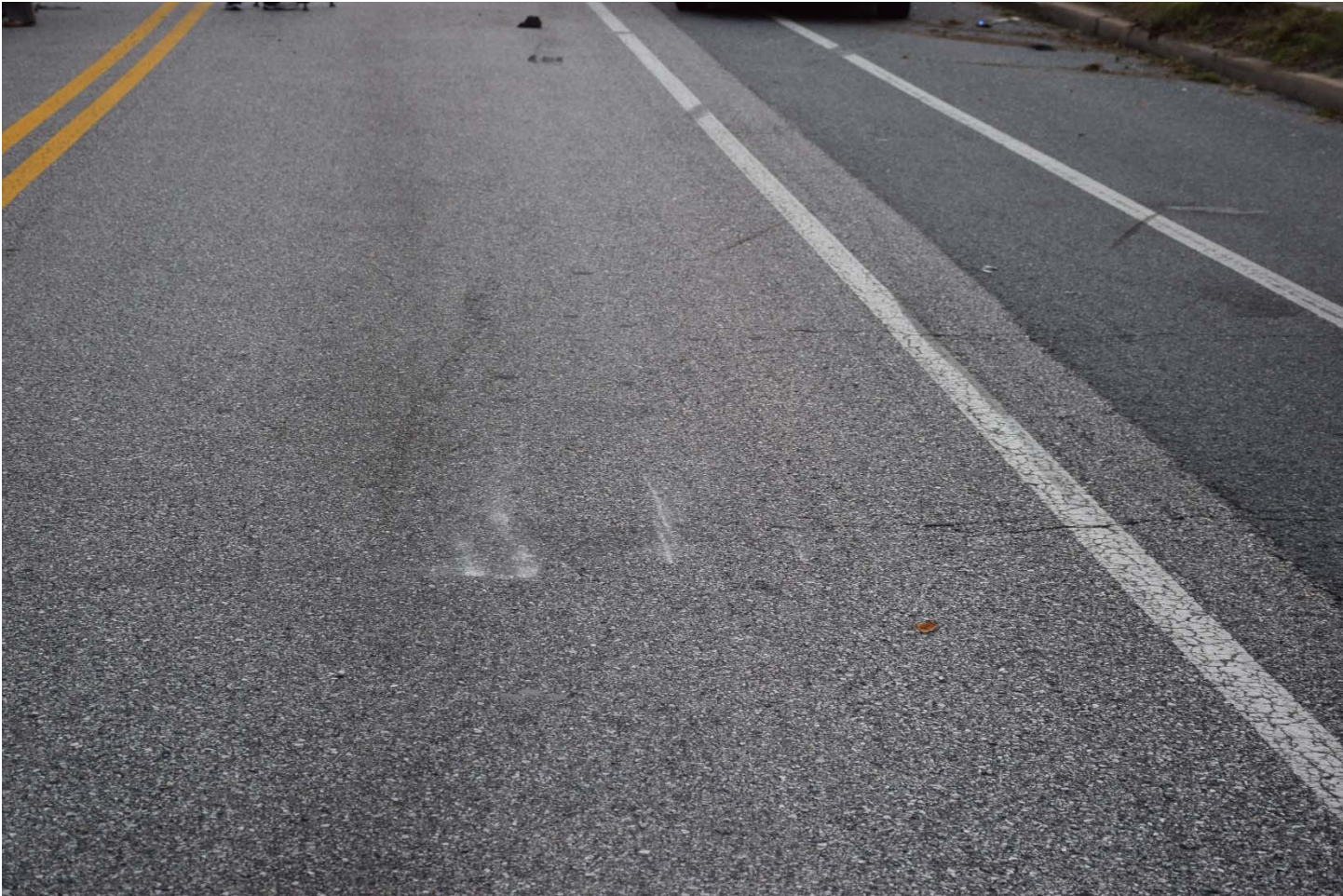
Highway Photo 3 – View of gouges and scrapes in pavement on Frederick Ave. where the school bus struck the rear of the Mustang.
