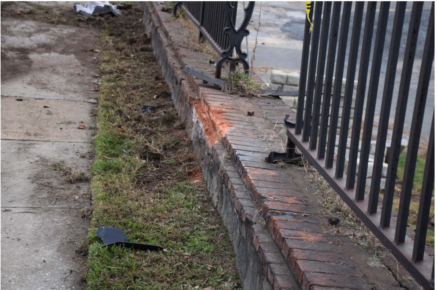
Highway Photo 16 – Close-up view of damage to cemetery wall from the Mustang’s secondary impact into the wall.
