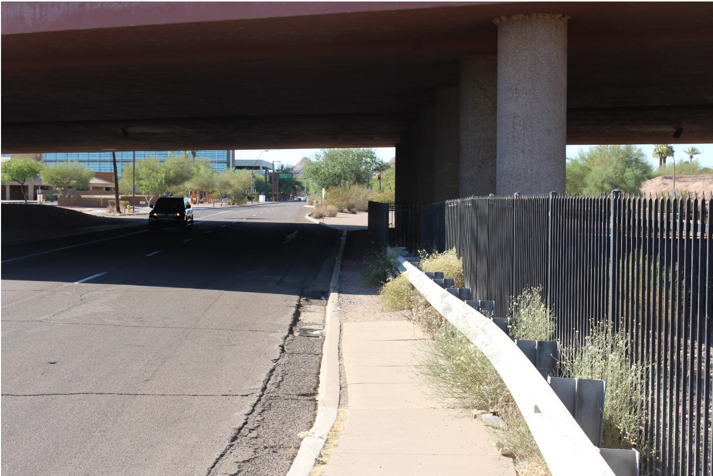
Highway Photo 1 – View of the pedestrian’s travel path into the median separating North and South Mill Avenue. Note the concrete sidewalk changes to a dirt path where the shadow of the overhead bridge begins in the photo.
