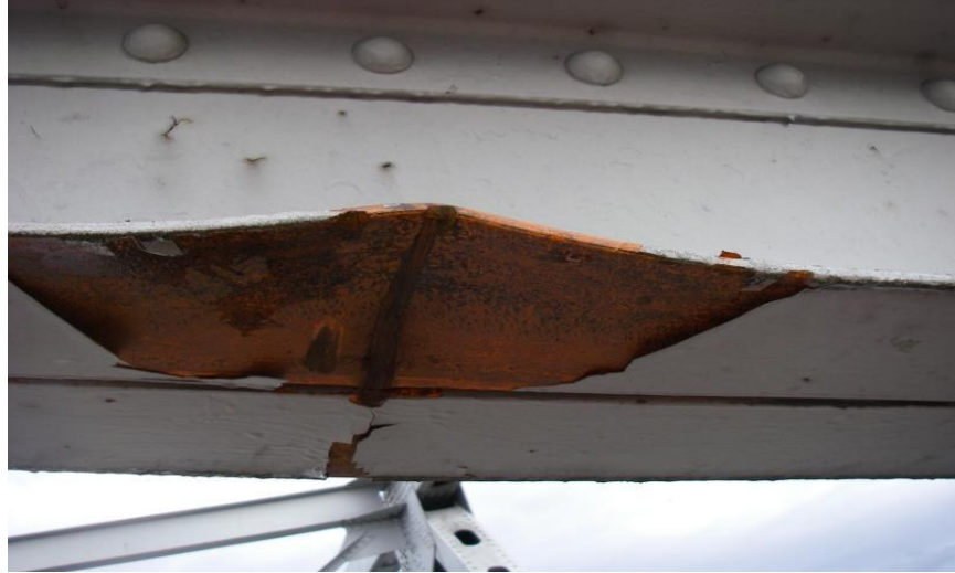
Photograph 4 – Damage to the U2 sway brace in Span 5 above the right lane in the northbound direction to the I-5 Bridge over the Skagit River as a result of the high load bridge hit on November 29, 2012
