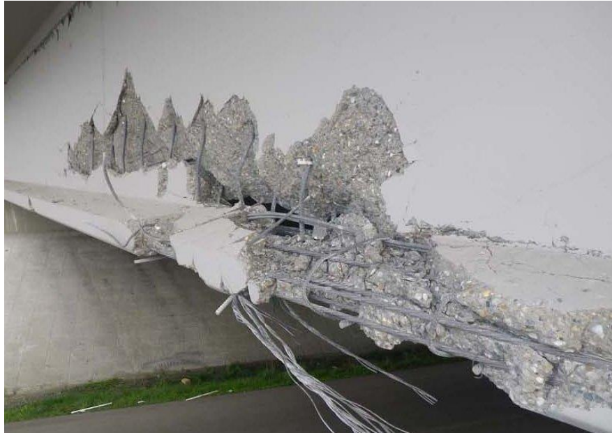
Photograph 5 – Damage to the State Road 16 and the Olympic Drive Overpass as a result of the high load bridge hit on March 17, 2013
