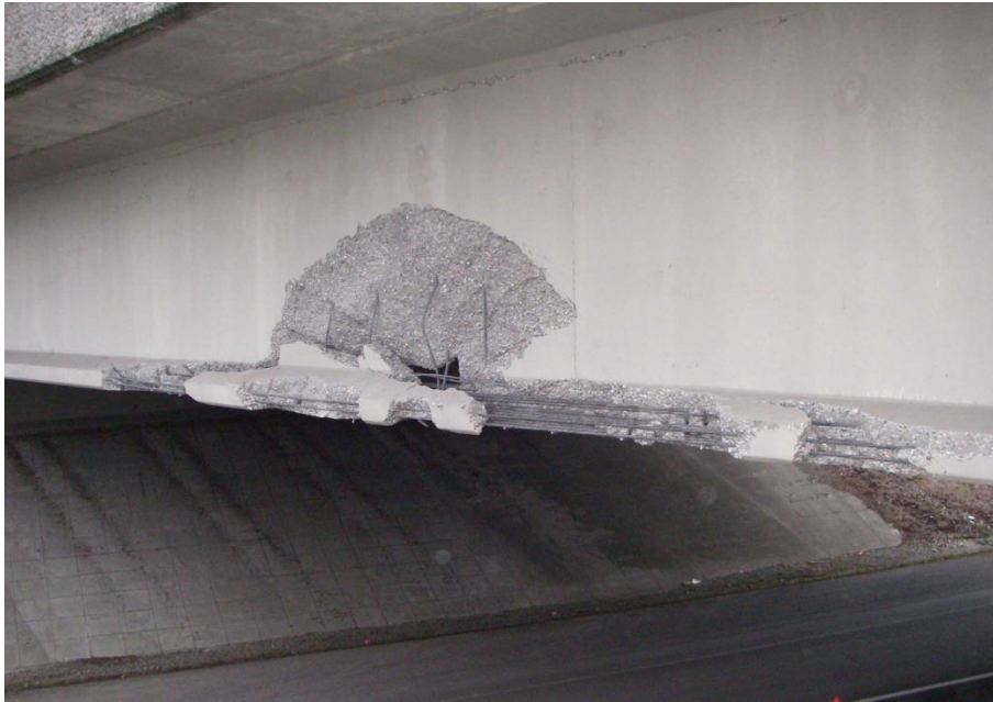
Photograph 6 – Damage to the State Road 16 and the Olympic Drive Overpass as a result of the high load bridge hit on January 4, 2011
