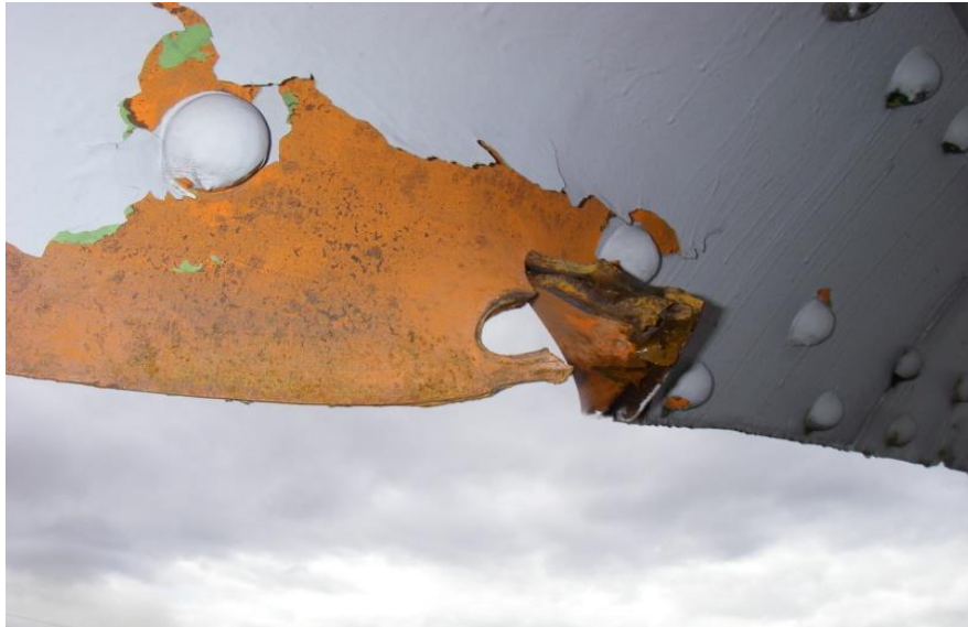
Photograph 3 – Damage to the U1 portal in Span 5 above the right lane in the northbound direction to the I-5 Bridge over the Skagit River as a result of the high load bridge hit on November 29, 2012
