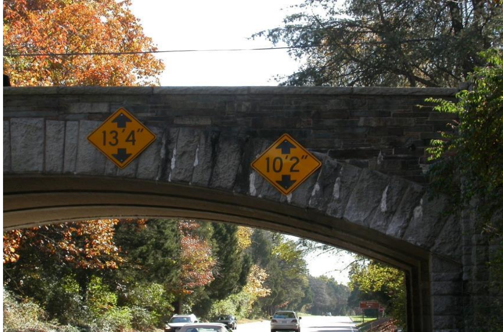
Photograph 9 – MUTCD low clearance signs (W12-2) that existed prior to the accident placed on the Alexandria Avenue Bridge Overpass face over the left and right lanes in Alexandria, VA
