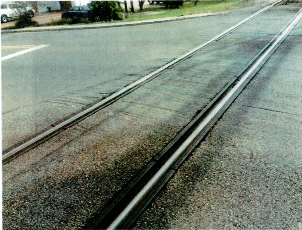
8. Iberville Dr.: Low clearance scrapes with a 17-foot span of overlay pavement.
