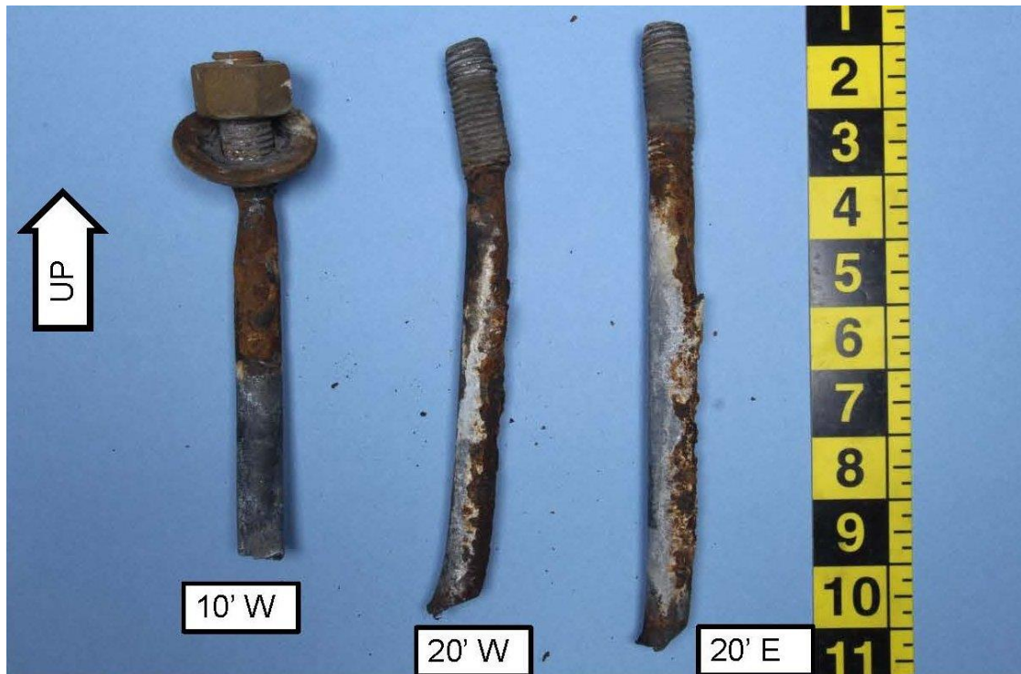
Figure 7. Pieces of U-bolt removed from the concrete parapet near where the HISD school bus surmounted the bridge rail.
