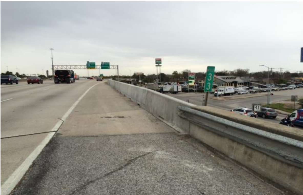
Figure 8. Looking to the southeast along the new single-sloped concrete traffic rail installed by the TxDOT Houston District after the crash. (Source: TxDOT Houston District)
