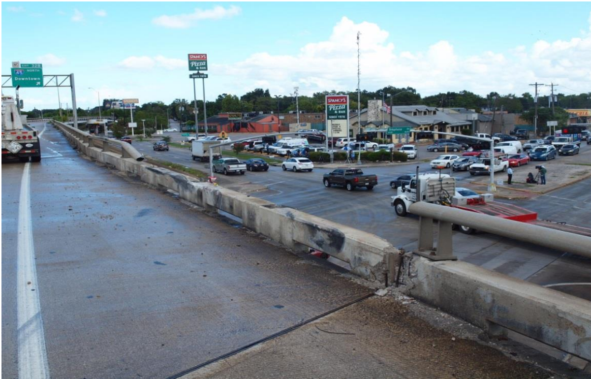
Figure 3. Bridge rail after being struck by the HISD school bus (view is to the southeast).
