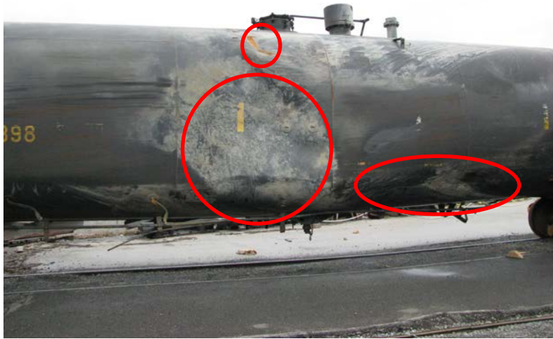
Figure 4: Three dents (highlighted in red) found on the left side of tank car UTLX 207398.
