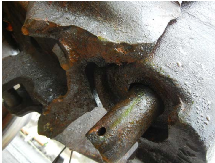
Figure 16: Another view of broken bottom shelf of A-end SE60EE double-shelf coupler on tank car OCPX 80323.
